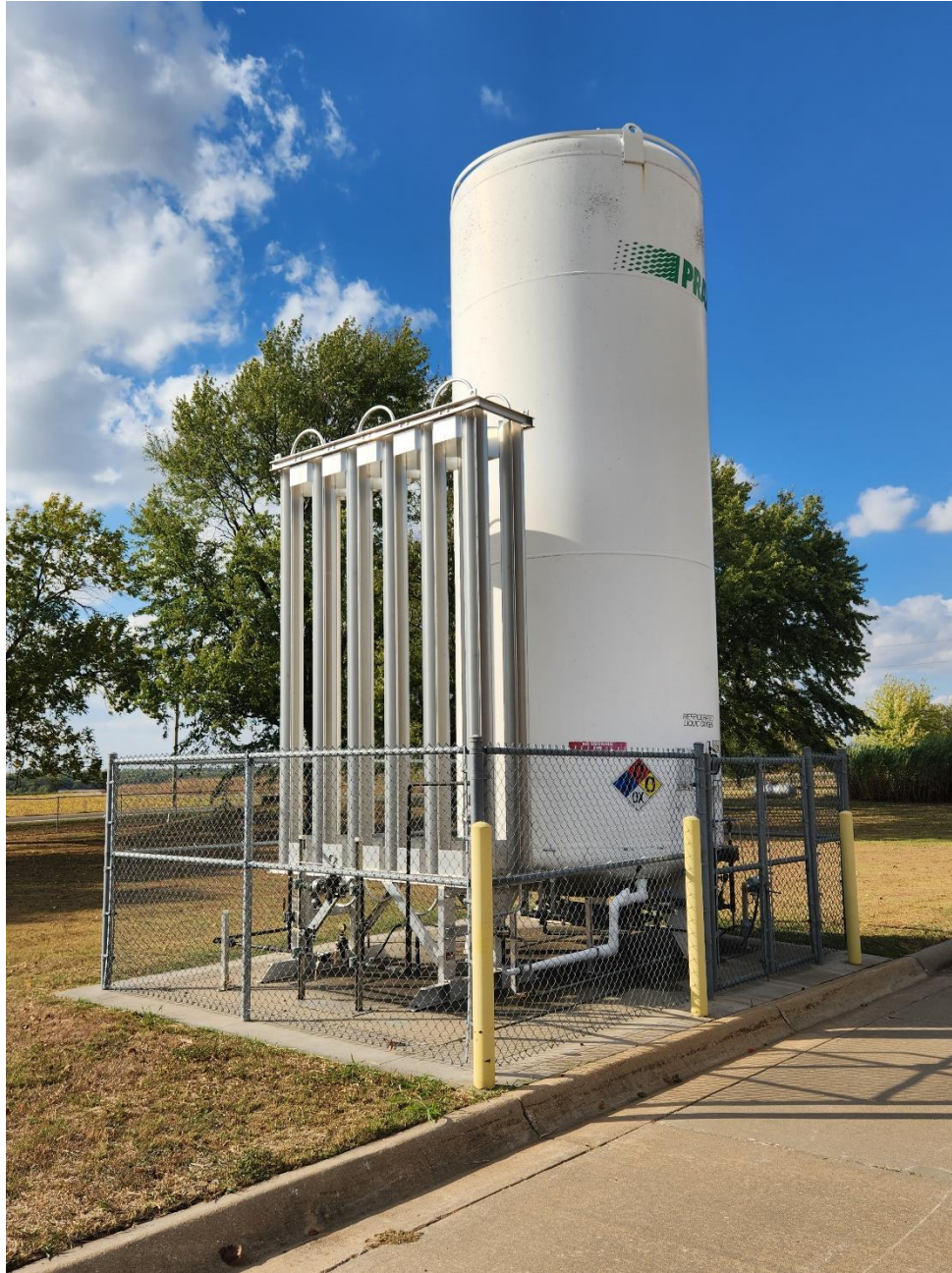
Figure 2: Liquid Oxygen Tank
