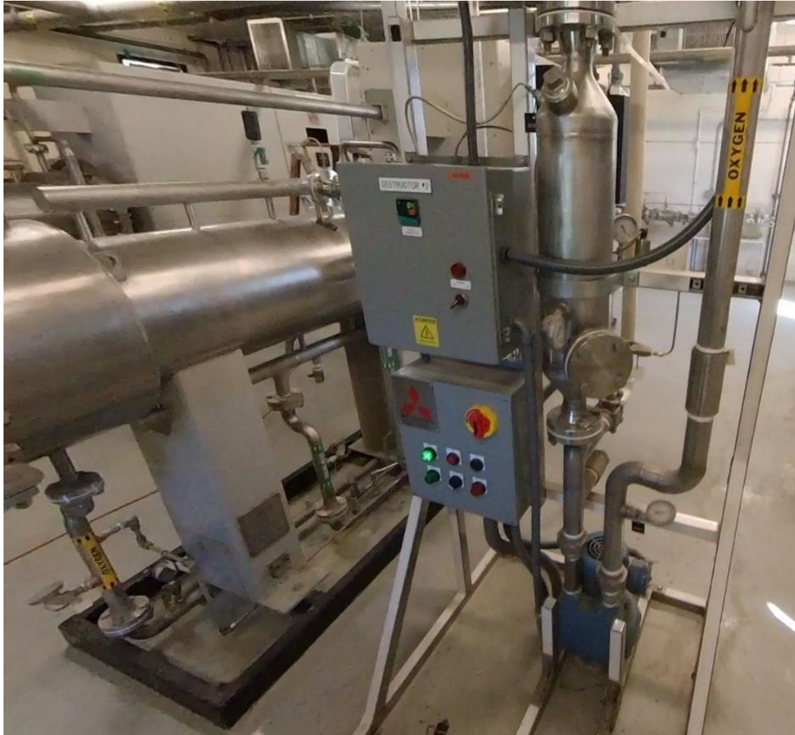
Figure 6: Ozone Destruct Units
