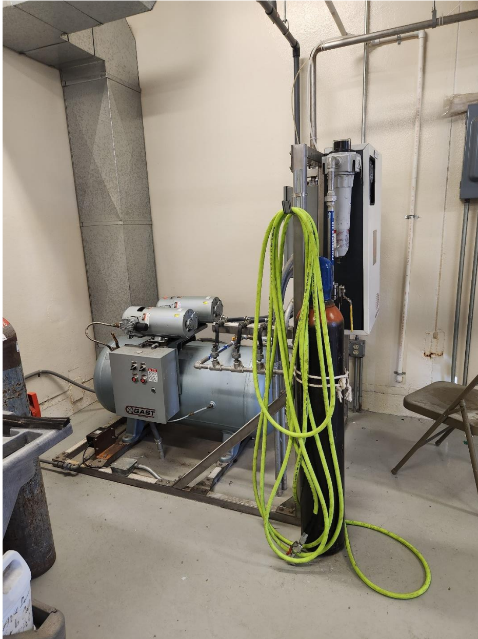
Figure 5: Nitrogen Boost System
