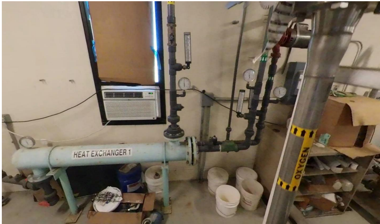
Figure 4: Mechanical Heat Exchangers
