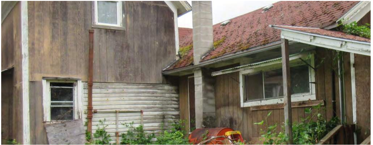
Figure 3: The image above depicts the current condition of the southeastern critical area as a result of continuous water infiltration. The increased growth of moss, warped shiplap siding, and joint where a cornerboard used to be are shown.
