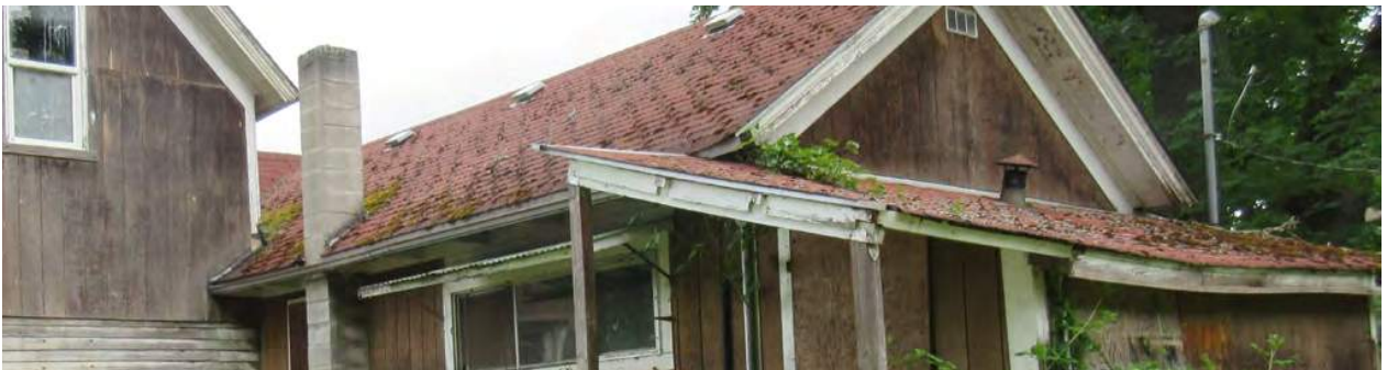
Figure 13: The three images above depict the amount of moss that has grown on the roof of the eastern façade of the 1890's kitchen addition (top), the northern façade of the garage and garage shed addition (middle), and the southeastern critical roof area as well as the roof of the 1890's kitchen shed addition (bottom).
