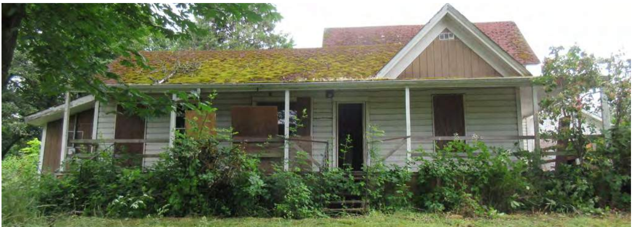
Figure 8 (before; after): The first image of the Briggs House above (top) exhibits the eastern façade in 2010 at the time of the UO assessment report, and the few handrails that were attached. The second image (bottom) exhibits the same façade in a poorer state seven years later. This image also displays the great amount of moss that has accumulated on top of the roof on this façade since 2010, as well as the placement of more temporary handrails.
