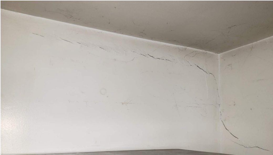
Un-repaired Horizontal cracking. Another example of the building walls being dragged during settlement event.
