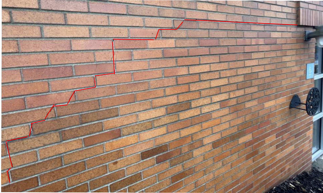
Horizontal and stepping crack (highlighted in red). This cracking is an example of the building being dragged during settlement event
