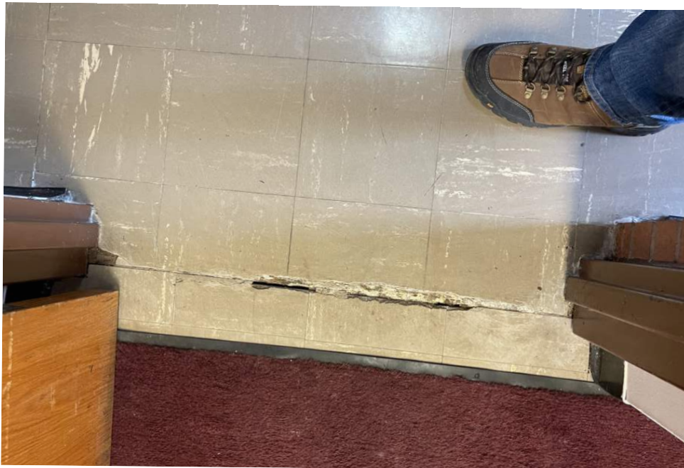
Un-repaired floor cracking. Crack is an occurred during settlement event.
