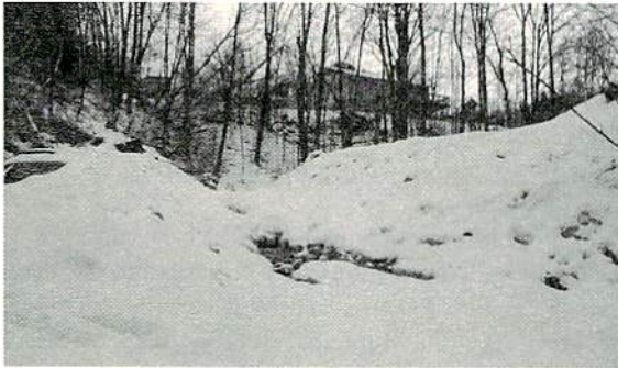
This temporary open channel replaces the 36" culvert and closes Sterling Hill Road.
