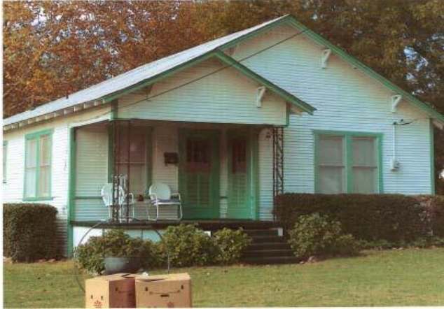
This porch has experienced an inappropriate alteration; wrought iron supports have replaced wood piers.
