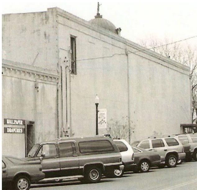
The upper-story windows on the side of this historic commercial building have been filled in with brick. Where instances like this exist, consider reopening the windows.
