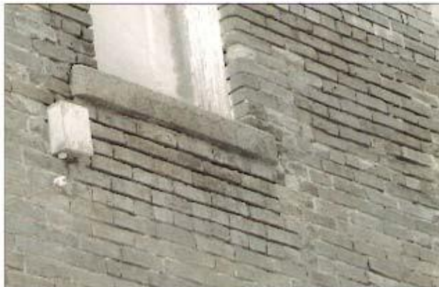
Protect masonry from water deterioration.
