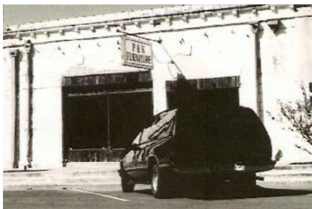
Although a storefront-like display window has been installed on this building, by altering the character of the original arched openings this building's historic integrity has been diminished.
