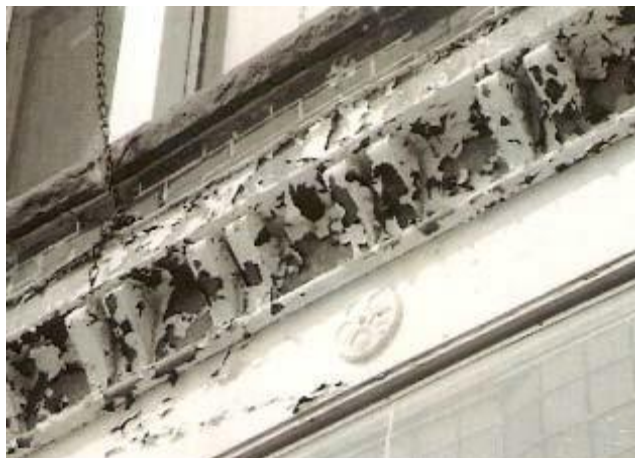
Maintain protective coatings, such as paint, on exposed metals.
