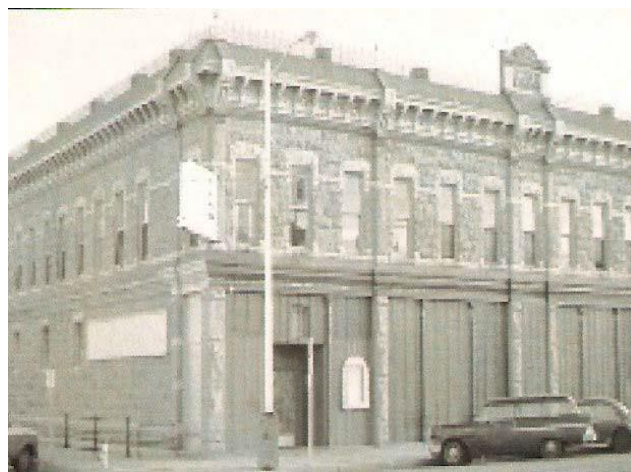
The windows in the structure were boarded and architectural details needed repair. (Compare with the photo below.)
