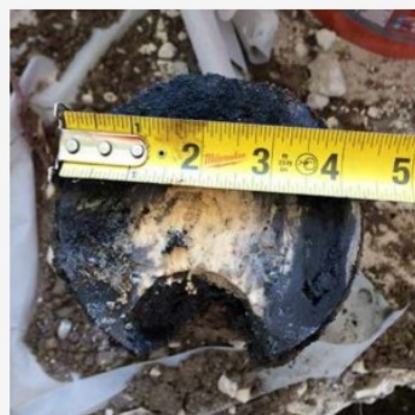
Figure A – Top view of a section of 4 inch cast iron pipe from a condominium experiencing severe FOG buildup.
