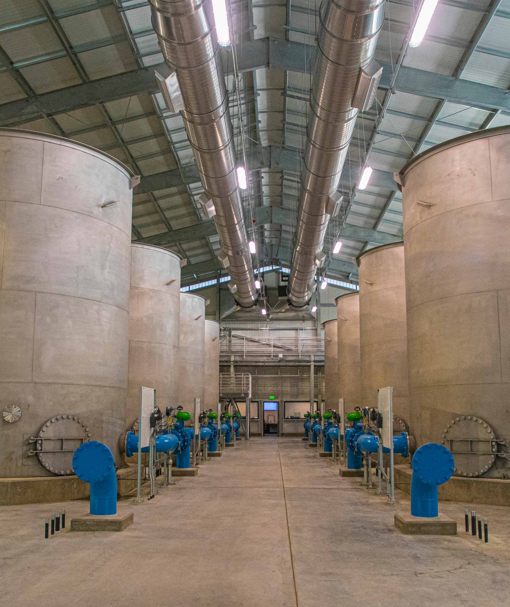
Ennis Water Softening Facility
