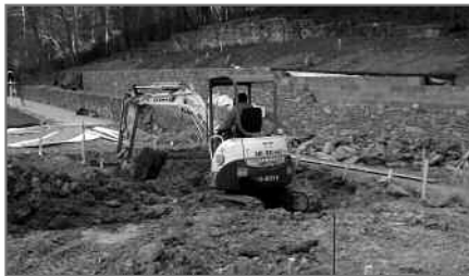
Excavation for New Baby Pool Being Built with a "Beach Entrance" for Easier Access.
