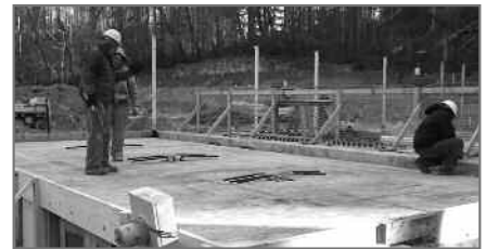
Framing to Replace the New Concrete Slab that Failed Under the Old Women's Bathroom.
