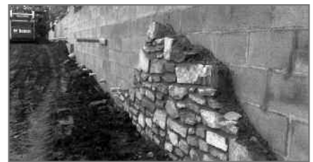
Mock-up of Stone Samples for Facing the New Retaining Wall Along the Expanded East Terrace.
