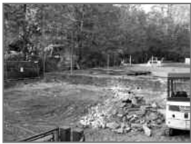
Baby Pool? What Baby Pool. Excavation on the New One Starts Soon.
