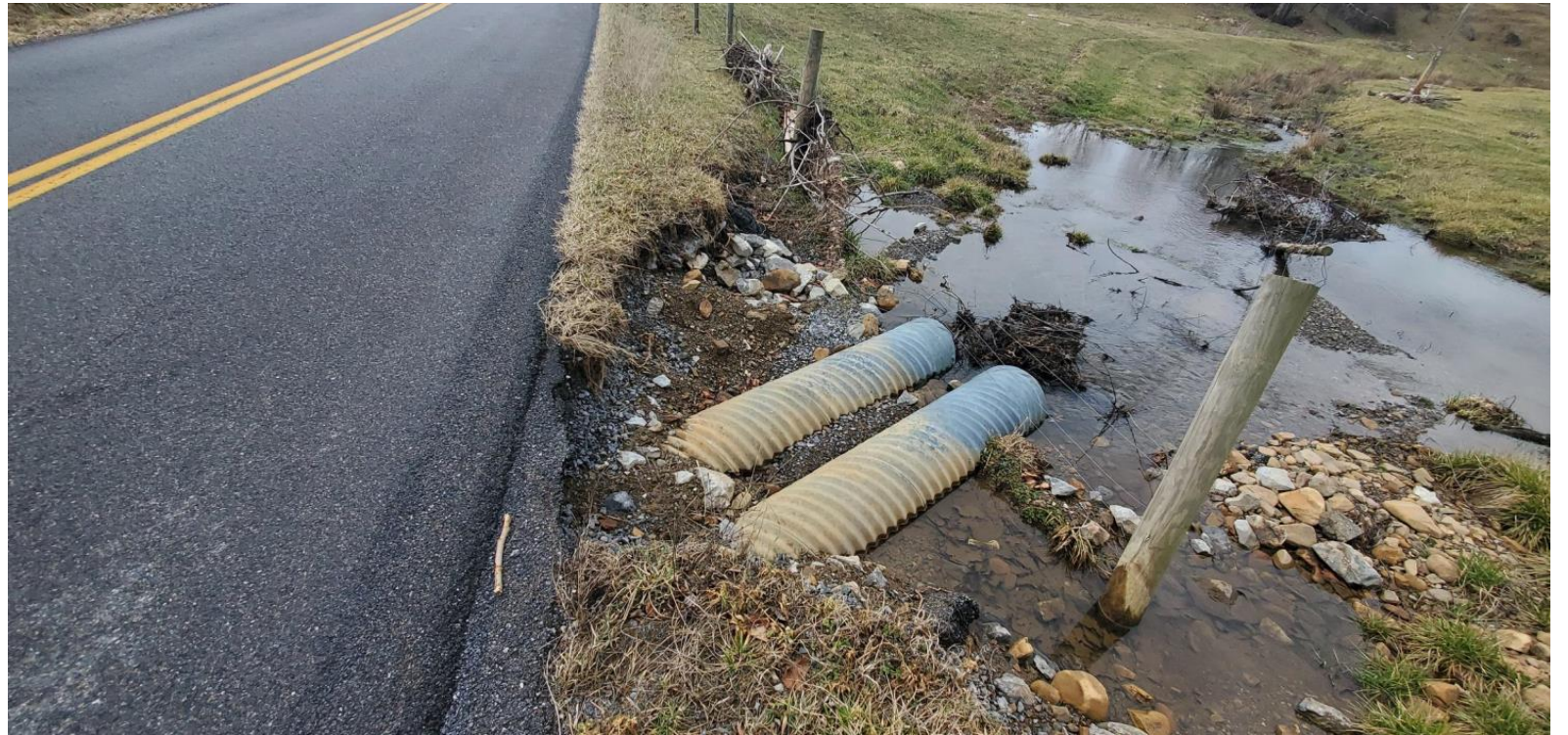
Roadway being undermined
