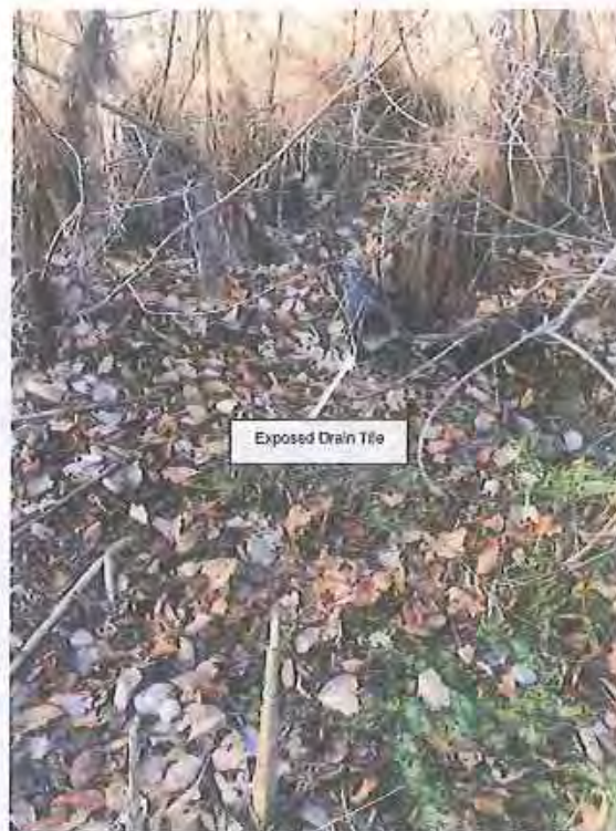
Photograph 4: Looking at southwest top of bank and exposed field tile entering pond.
