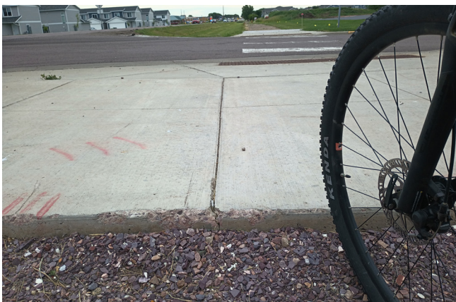
FIGURE 3.7 The unpaved path at the intersection of W Willow Street with Honeysuckle Drive has a vertical trip hazard where the unpaved and paved surfaces meet. This can be corrected by adding material to meet the level of the concrete surface.
