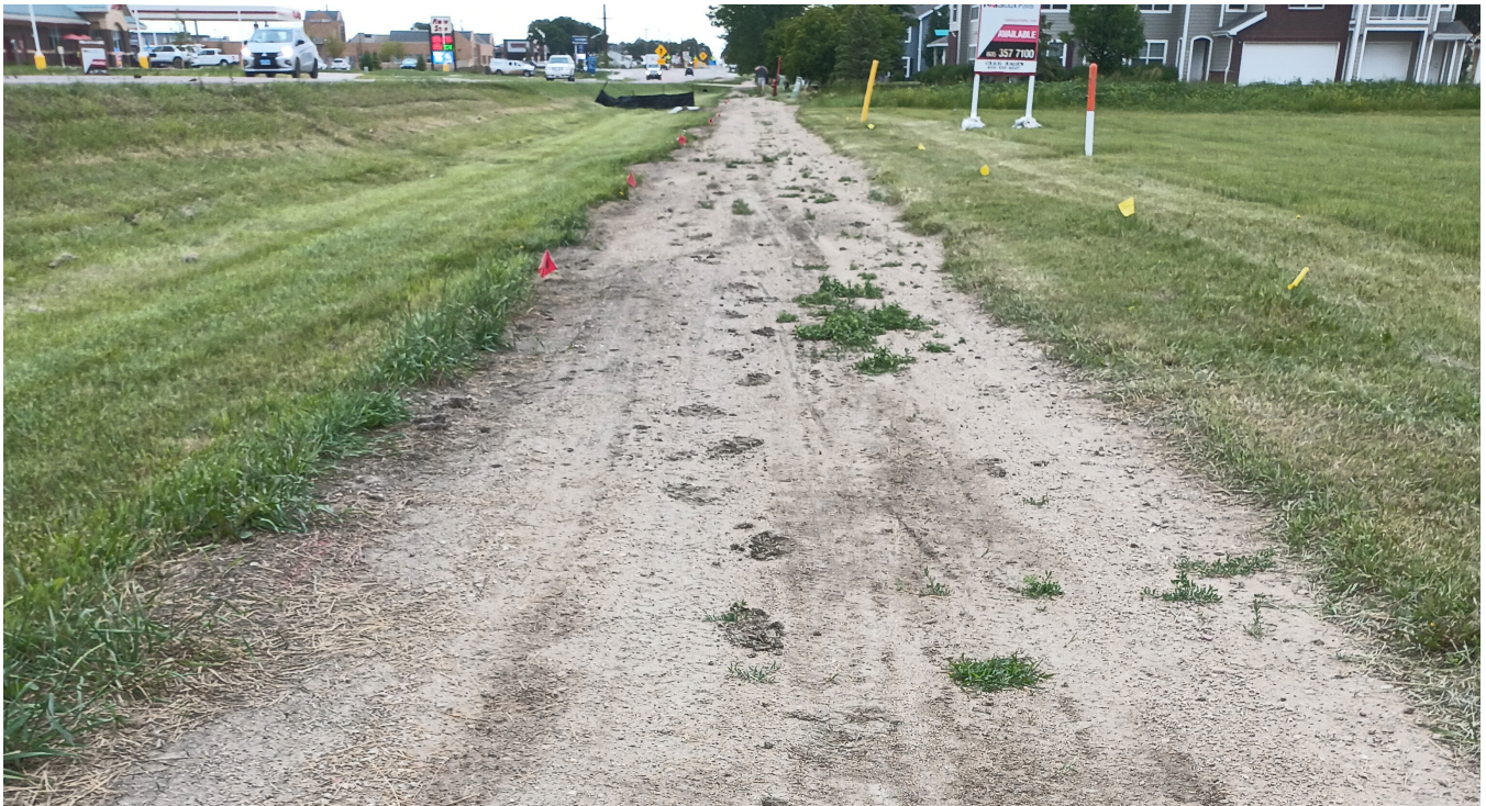
FIGURE 3.6 Footstep and bicycle wheel indentations can be seen on this segment of unpaved trail along Willow Street.
