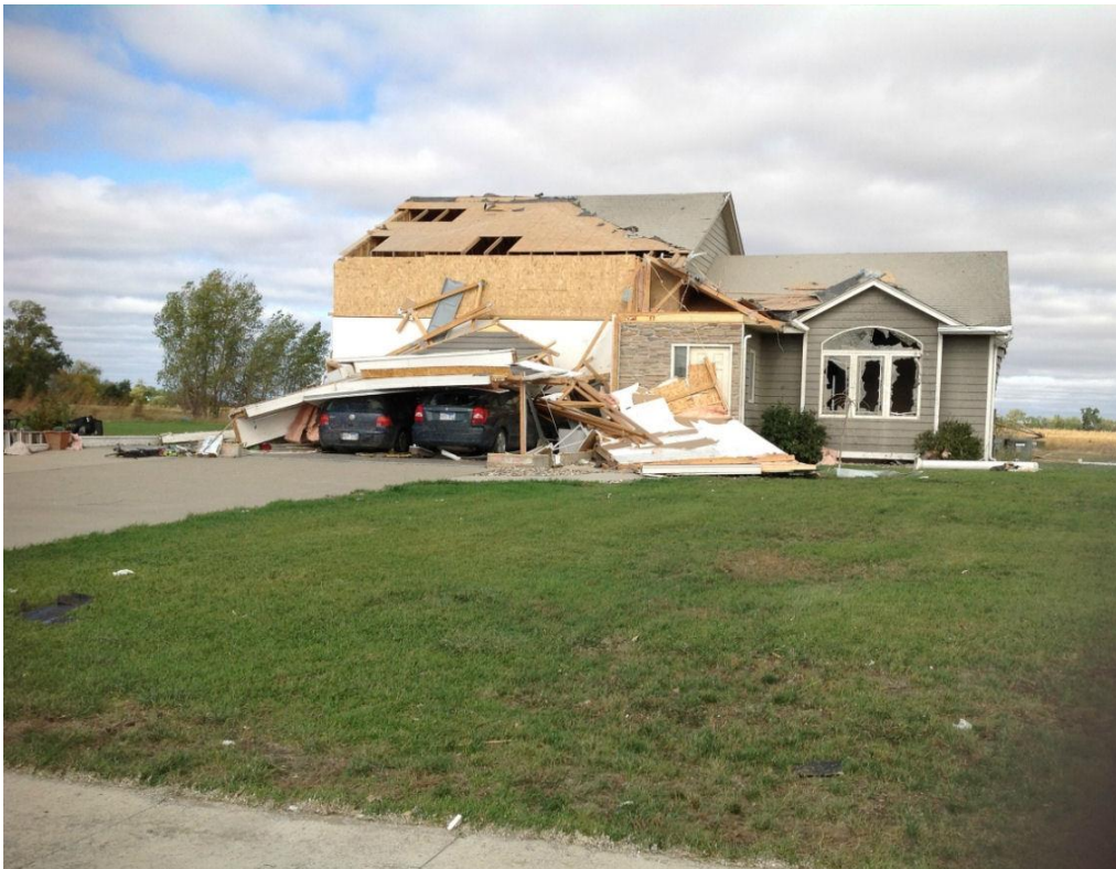
Tornado damage in McCook Lake, SD, National Weather Service, October 4, 2013
