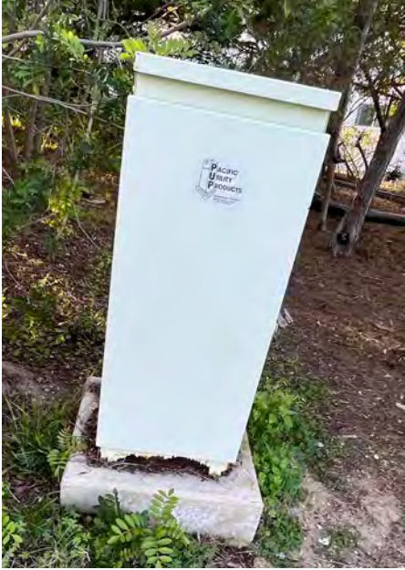
Figure 13: Corrosion rotted irrigation electrical box
