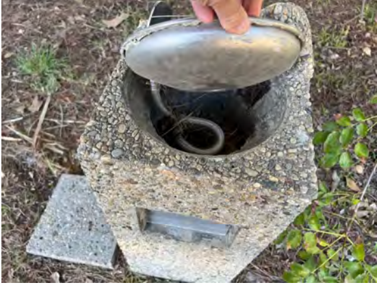
Figure 14: Water fountain bowl loose and drain is gone
