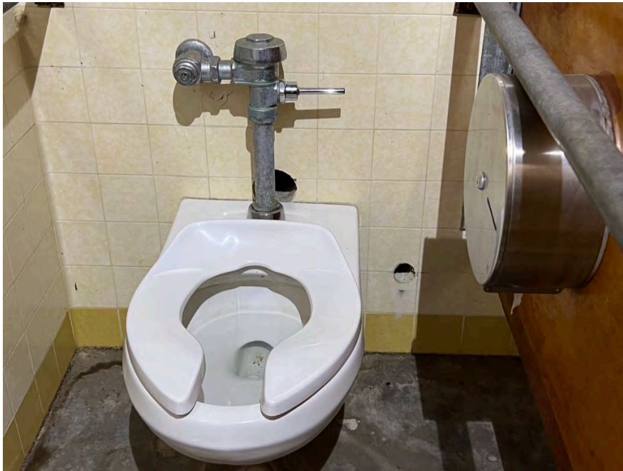
Figure 22: Not very clean feeling, exposed holes in wall
