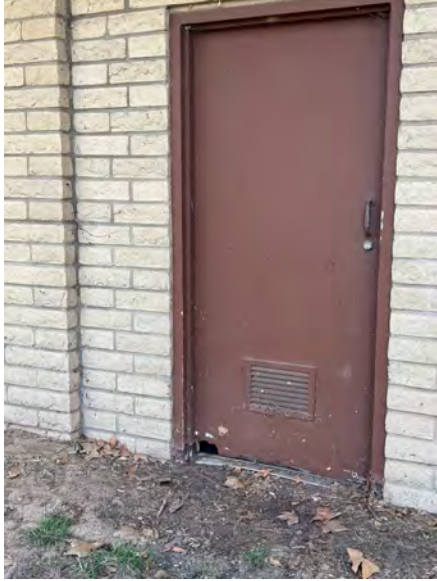
Figure 21: Rodent chewed hole in door of maintenance area of restroom
