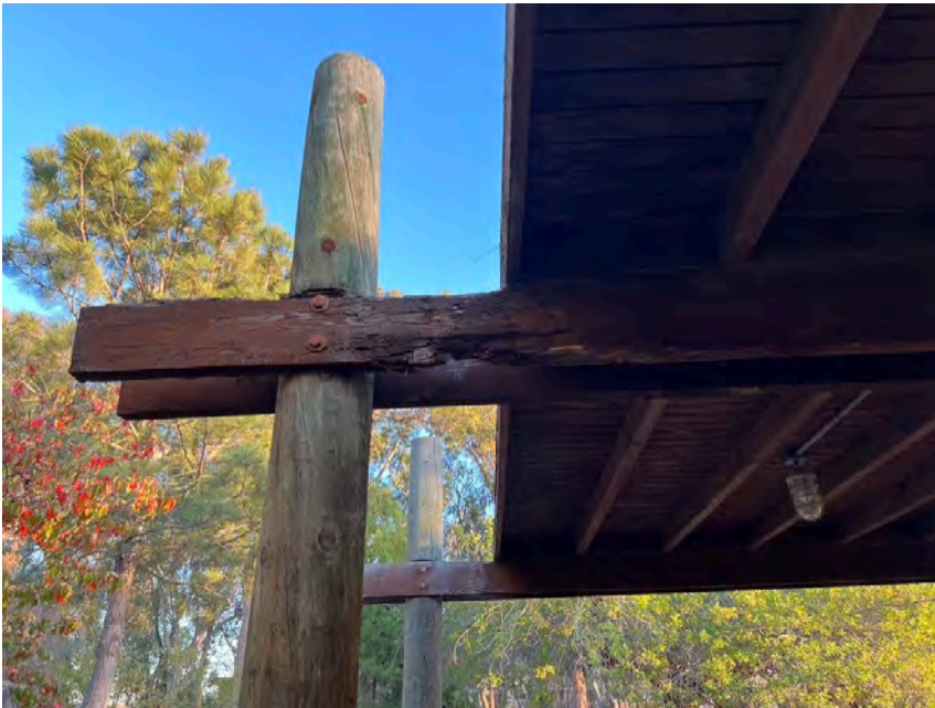
Figure 15: Rotting support beams on Community Center
