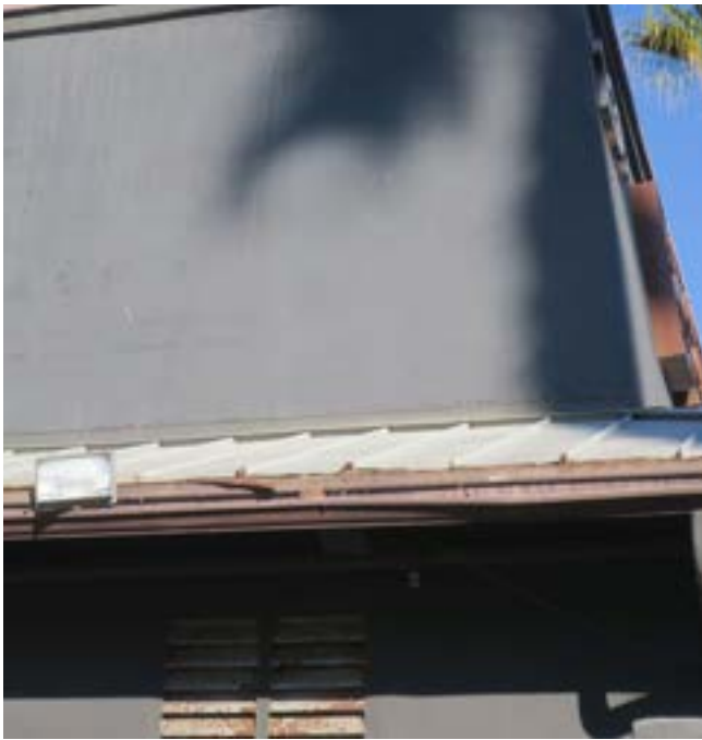
Localized corrosion (rust) at standing seam roofing
