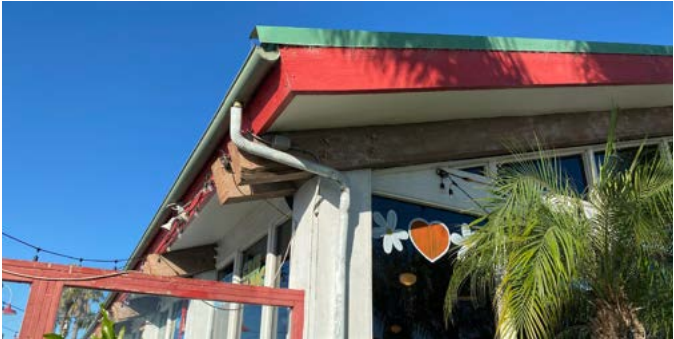
Downspout disconnected from gutter
