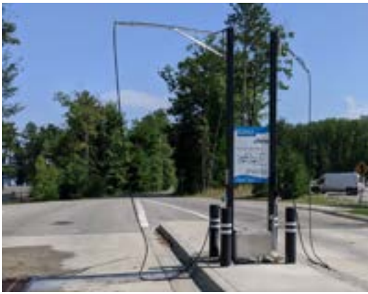
Boat wash station
