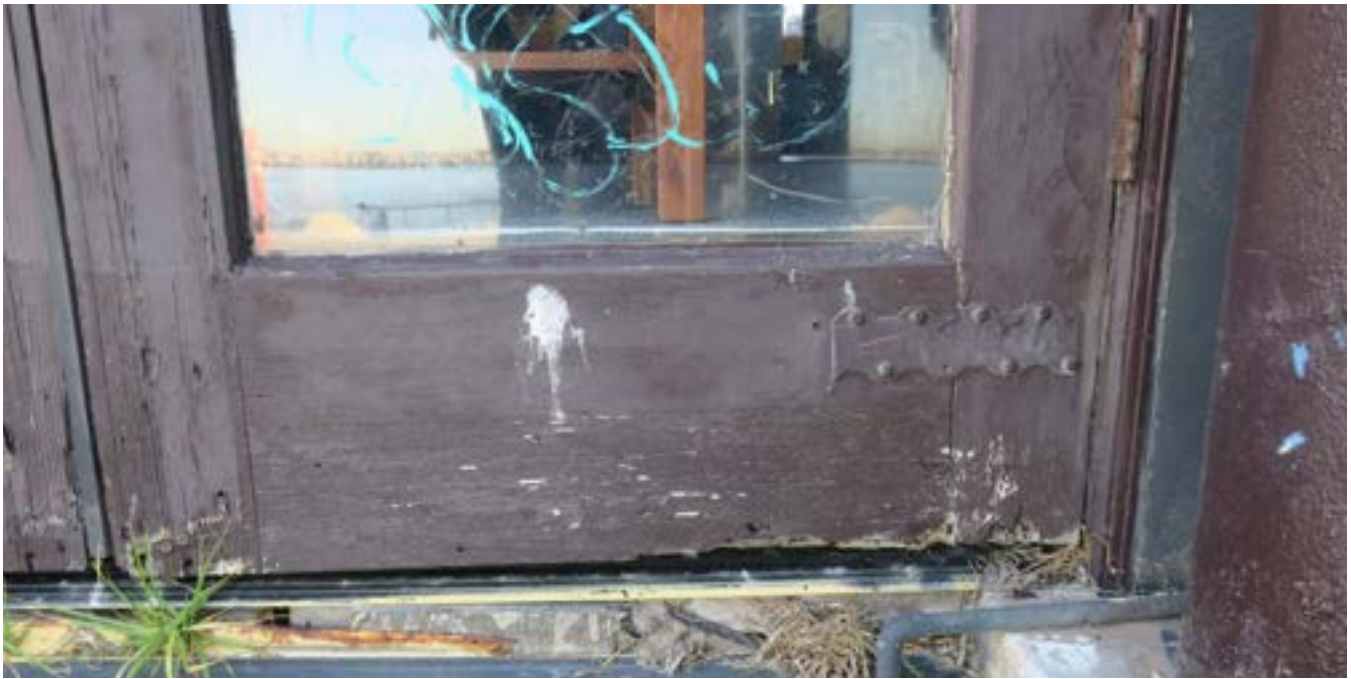
Wood decay and deteriorated flashing at base of doors
