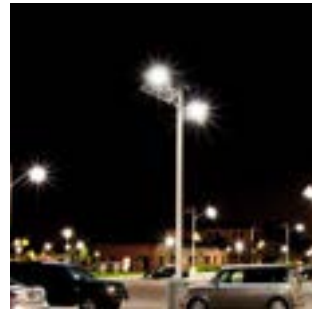
Parking lot lighting
