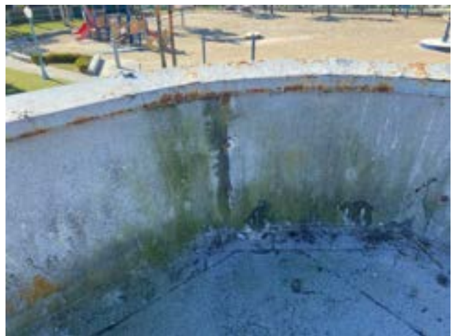
Bio growth at roof-side of parapet walls
