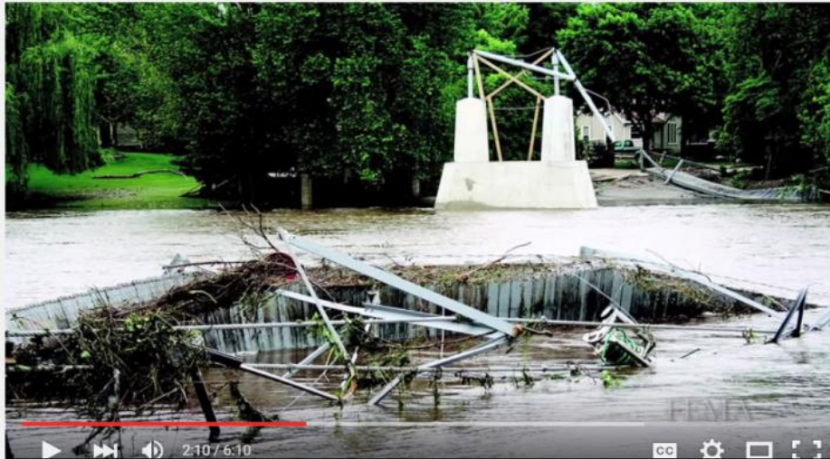
Pedestrian Bridge Remains After 2008 Flood
