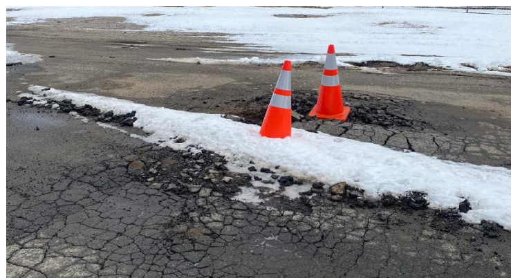
Internal roads in need of repair
