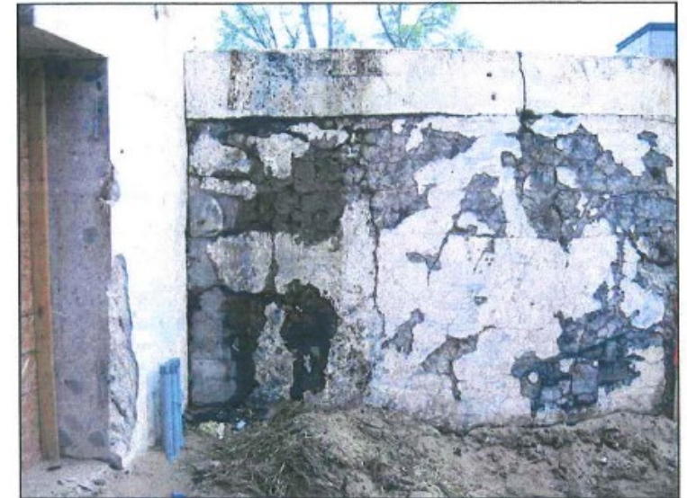
PHOTO NO. 3: West Wall - No Concrete Repairs
