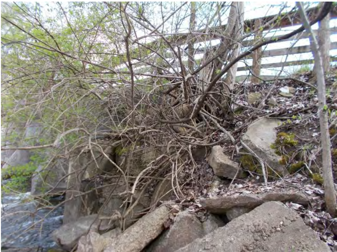
Tree and brush growth in northwest quadrant
