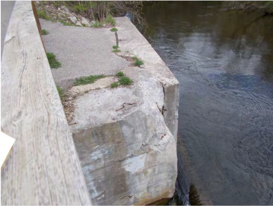
Spalling and prior repairs on southeast abutment/wingwall area
