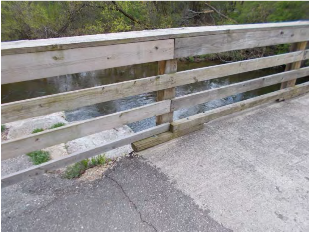
Weathering and splitting in timber railing
