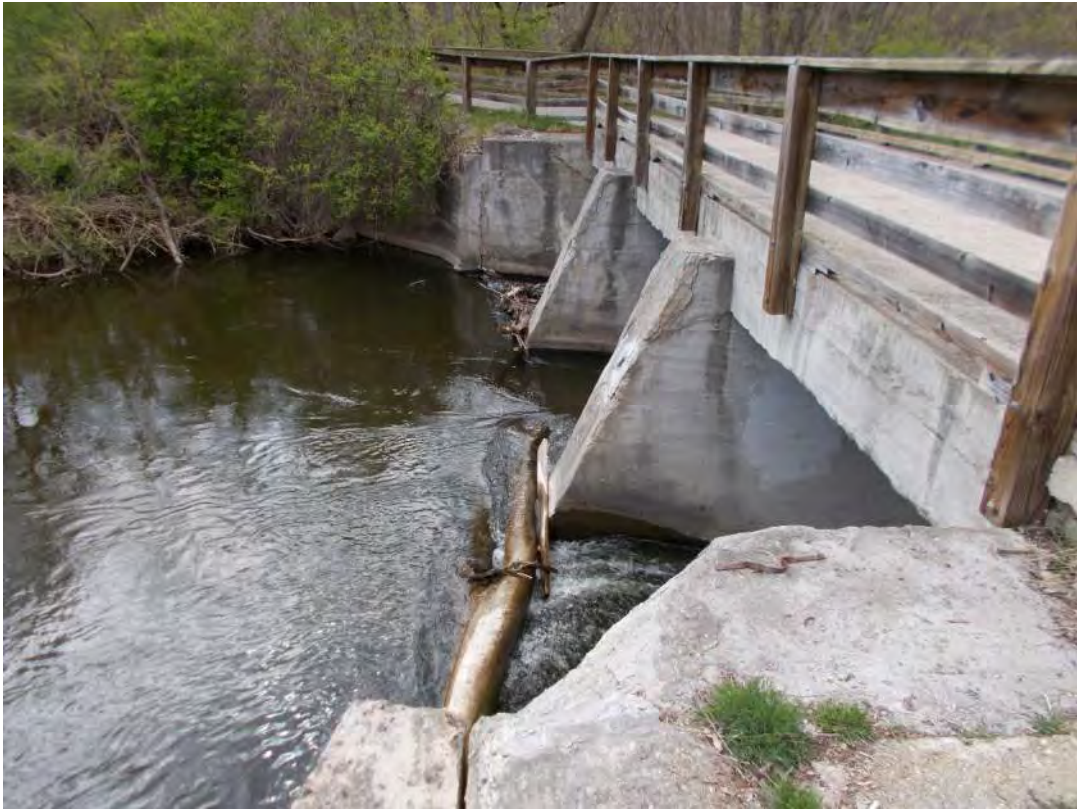
Heavy timber debris caught on piers
