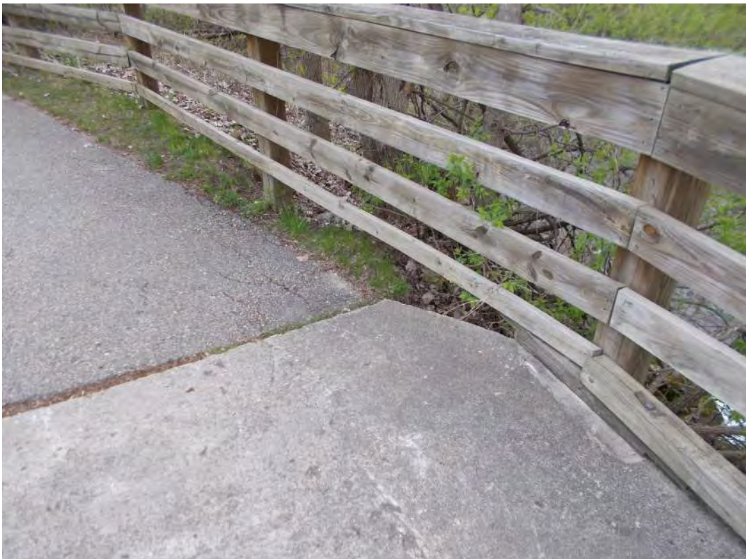
Slope erosion in northwest encroaching on trail
