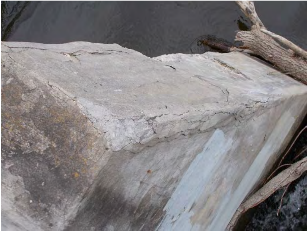
Cracking and delamination on south end of west pier
