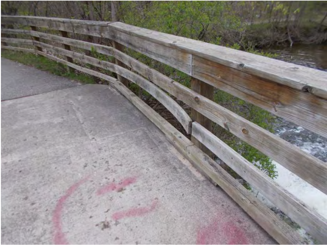
Severe warping in timber rail member in northwest
