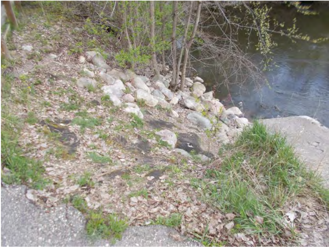
Exposed geotextile from riprap loss at end of southeast wingwall
