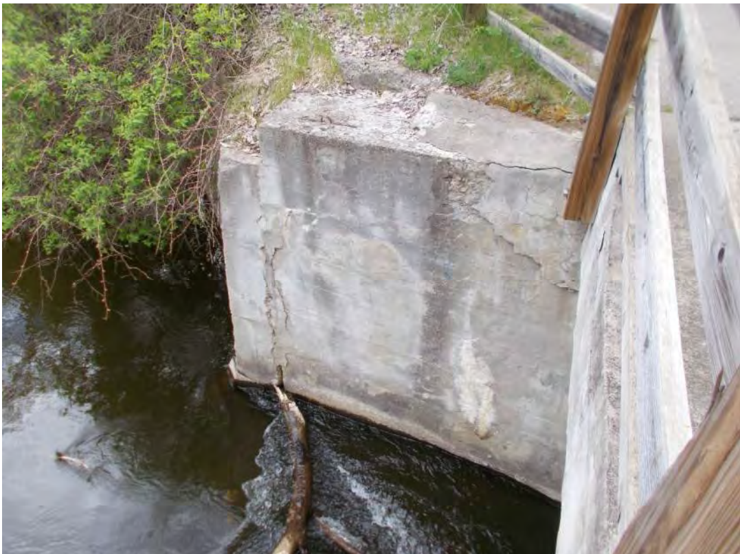
Cracking and delamination on southwest abutment/wingwall area
