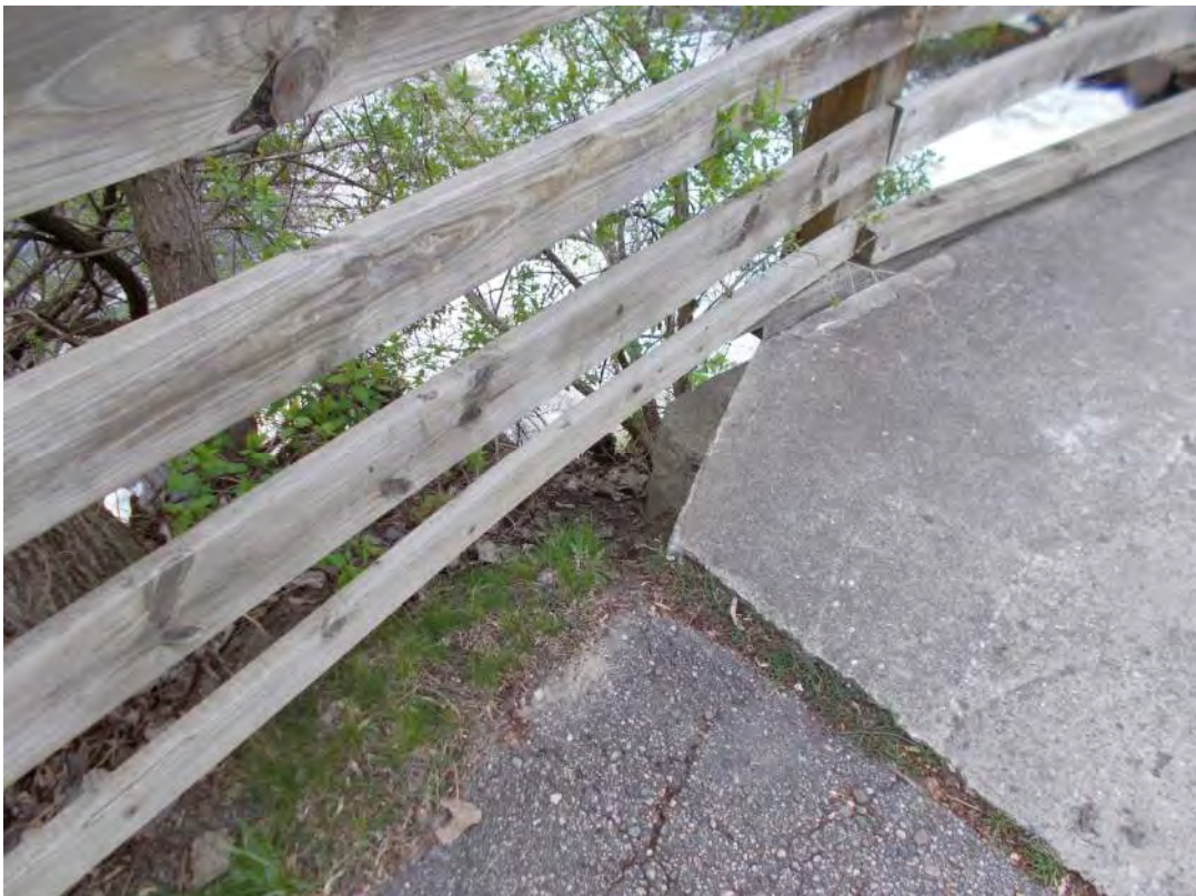
Slope erosion in northwest encroaching on trail
