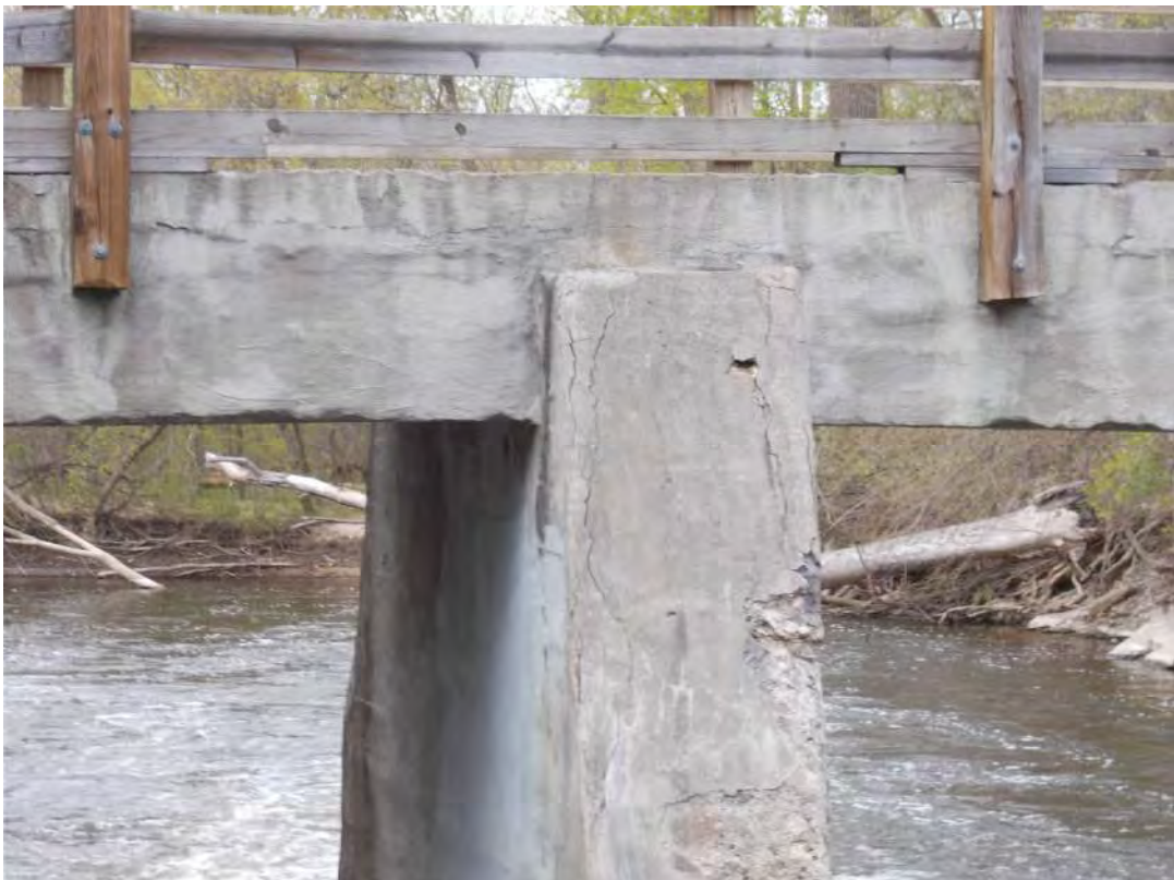
Cracking, delamination and spalling on upstream end of pier
