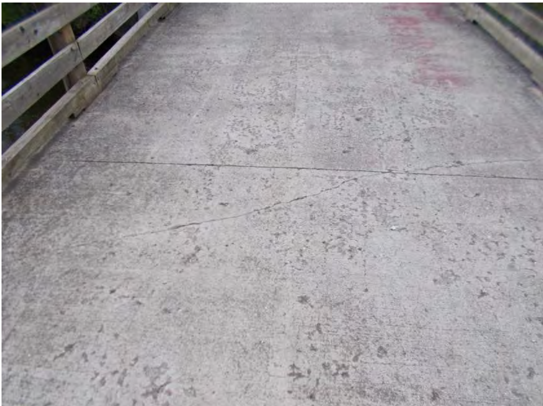
Cracking and scaling in concrete surface
