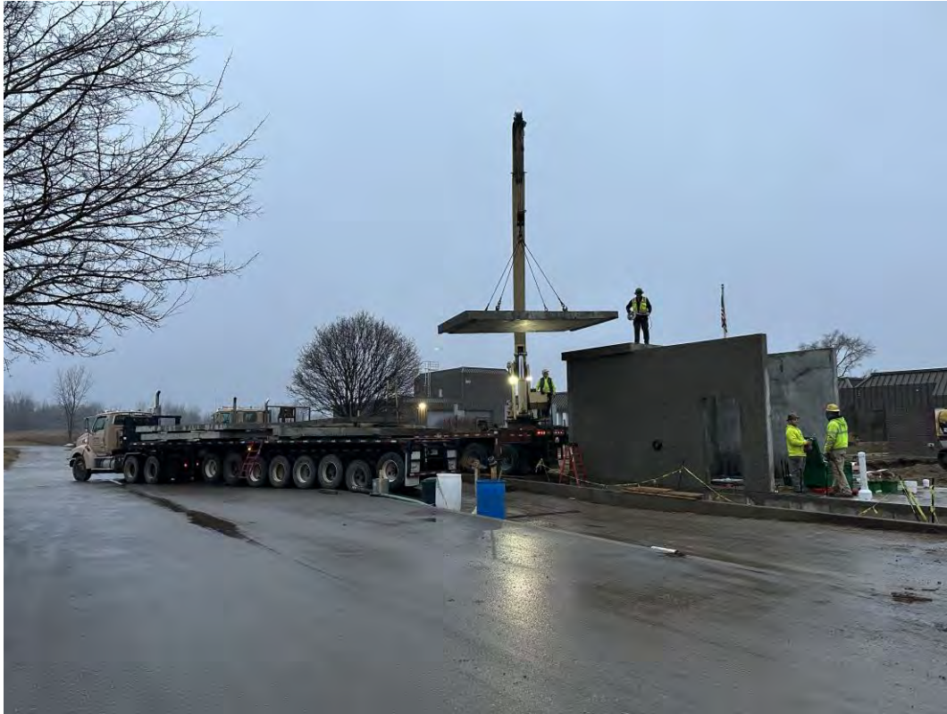
New Septage Receiving Building With New Card Swipe Payment System
