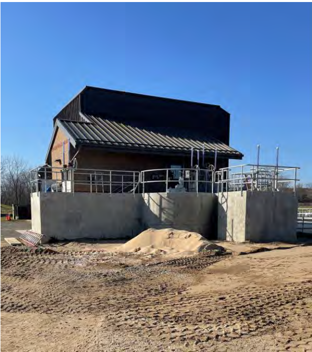
New grit building and grit vortices
