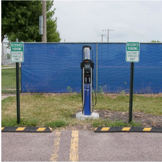
Figure 6-15. Caswell Park Sports Complex Electric Vehicle Charger.
