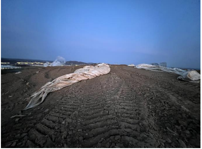
Photo 8: Unused tarps 80 feet from the active face.
