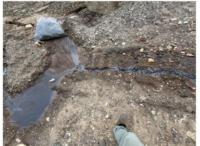
Photo 12: Second seep along road near photo 11.
