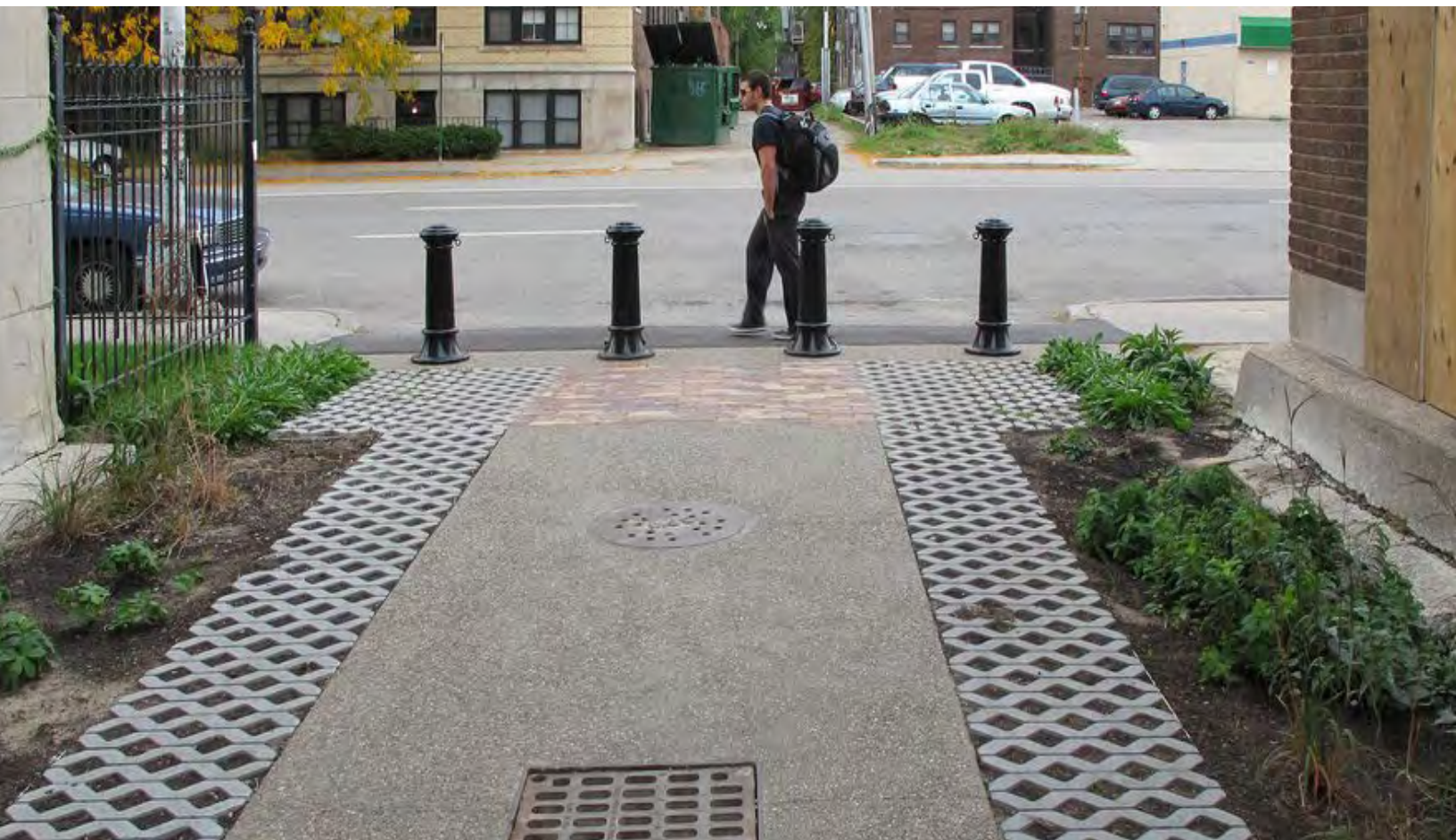
FIGURE 9.6 - EXAMPLE OF A GREEN ALLEY CONVERSION SHOWING BOTH REDUCED PAVEMENT AREAS AND POROUS PAVEMENT
