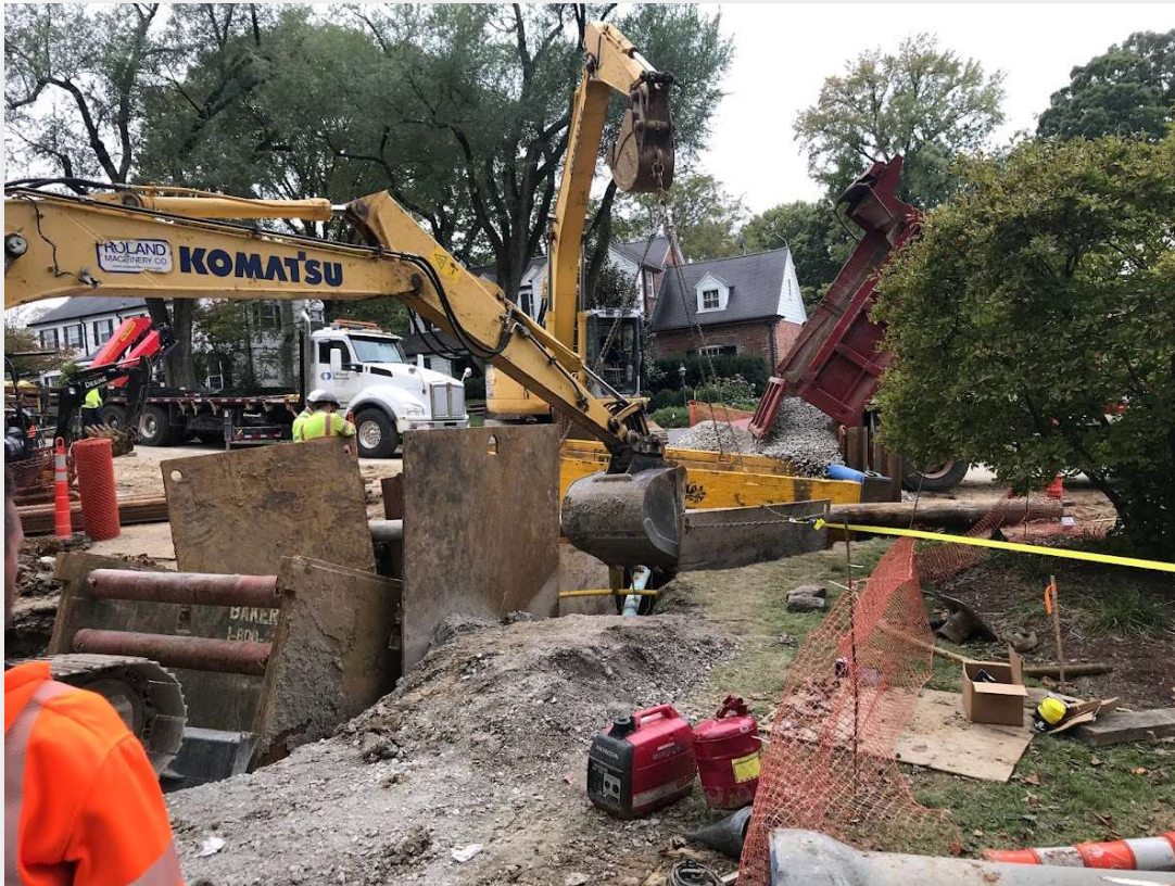
Figure 12: Construction of the Willow Hill Stormwater Infrastructure project posed several challenges, including the placement of new stormwater pipe in the vicinity of crisscrossing existing gas and water mains, all while navigating poor soil condition
