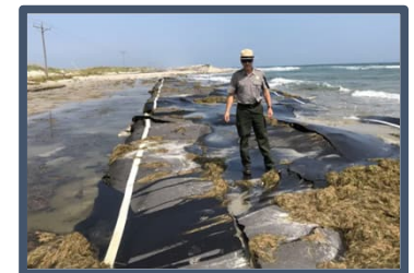
Superintendent David Hallac standing on a damaged stretch of NC-12 after Hurricane Dorian. Source: NPS
