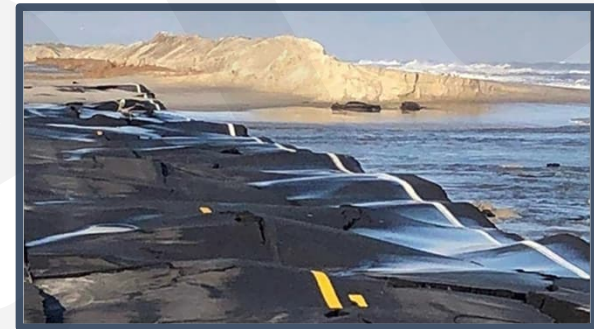
NC12 post Hurricane Dorian in 2019. Source: NCDOT
