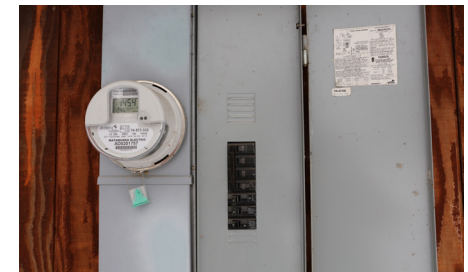
Meter and breakers
