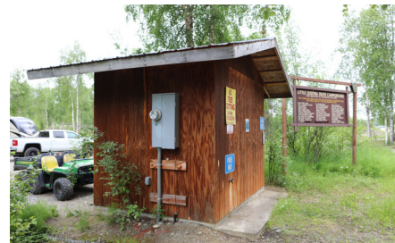
Water and power shed at camp host site
