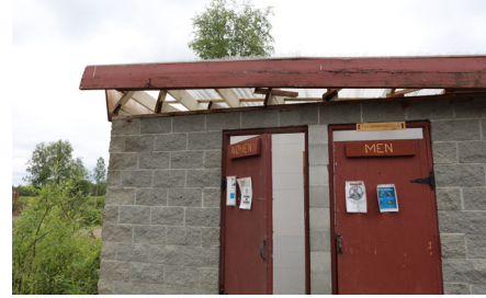
Vault toilet - western area
