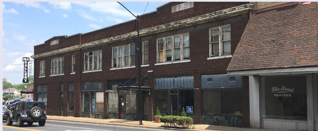
The Phoenix Building, located on one of Downtown's most significant corners - the intersection of Ninth and Main - should be a top priority for preservation and rehabilitation.
