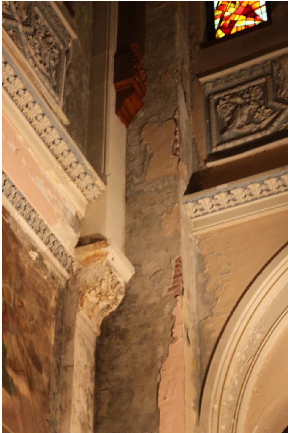
Missing Plaster at North Transept
