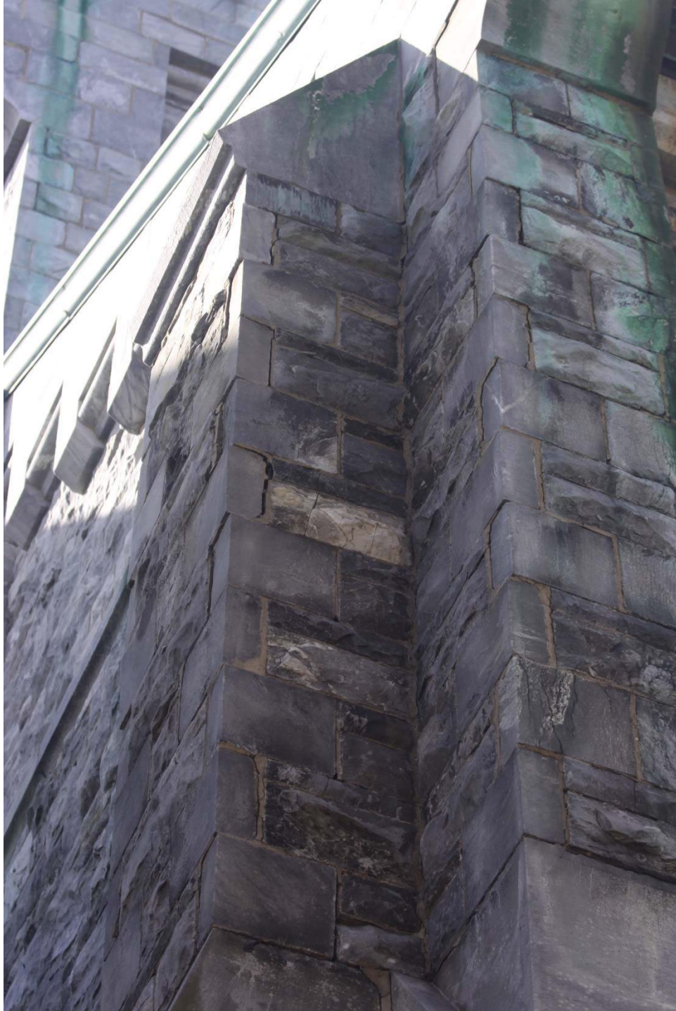
Exterior buttress of North Transept in need of repointing/repair
