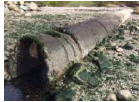
Photo of Mount Hope Avenue CSO Outfall looking east toward Atlantic Boulevard.
