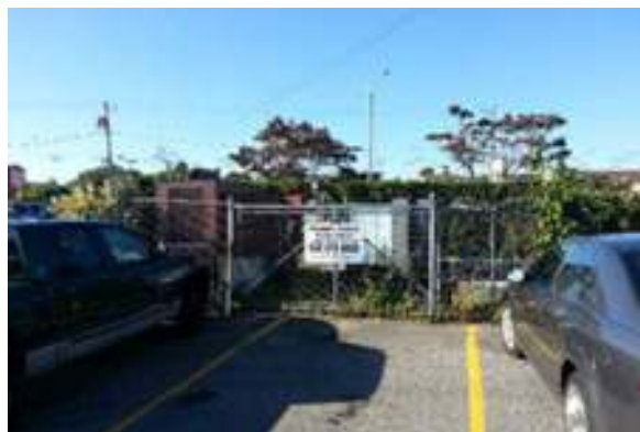
The President Avenue pump station is beyond its useful life and should be replaced as soon as possible. In 1981, the failing pump station wet well was retrofitted with submersible pumps—as a temporary solution. These pumps are still in service.
