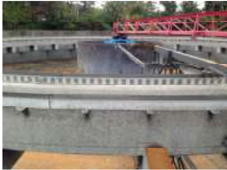
Clarifier No. 3 is out of service. The center drive cage sheared and requires replacement.
