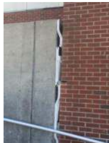
Settlement exhibited in building joint and stairs at Pump House No. 2. Settlement has resulted in piping and electrical service failures.
