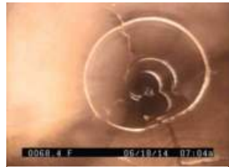
Closed-circuit television image showing a cracked pipe
