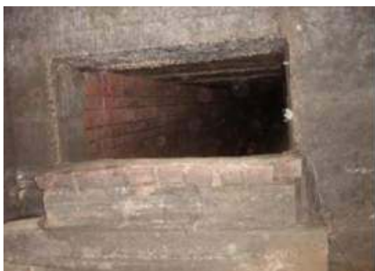
A view of the CSO weir and outfall pipe inside the Davol No. 2 CSO Regulator Structure.
