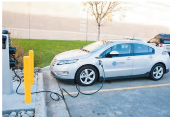
Electric charging station example
