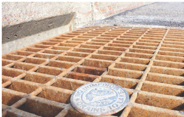
Example of storm water Drain
