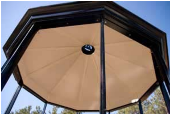
The lantern's ceiling as seen through the empty window casements.
