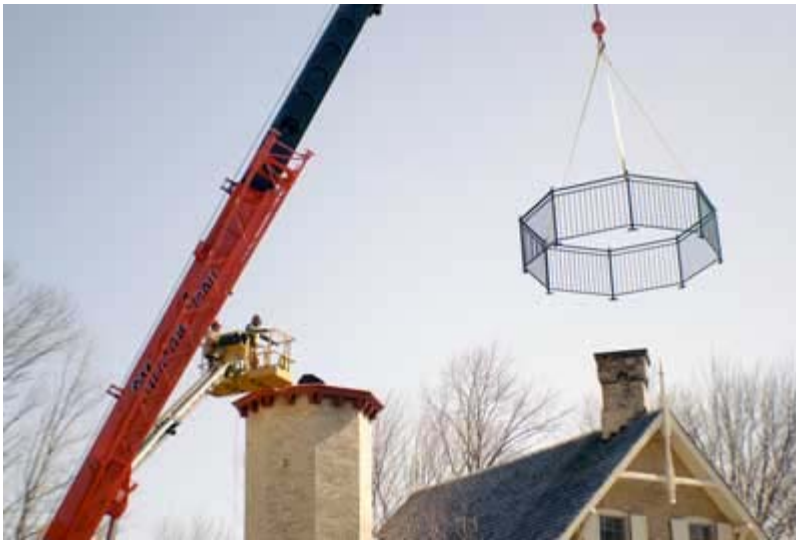
The railing is lifted into place, with installers in a cherry-picker directing the crane operator.
