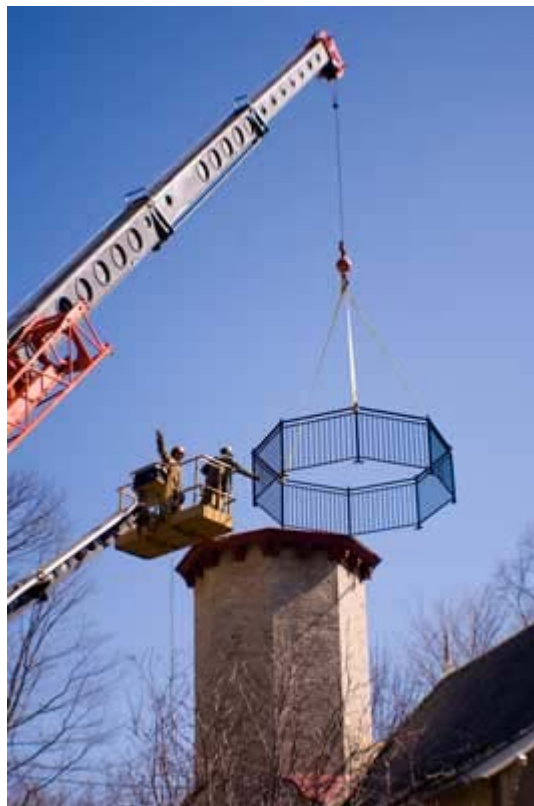
The railing is about to come to rest atop the lighthouse, where it will be secured by thick bolts to the 160-year-old tower .
