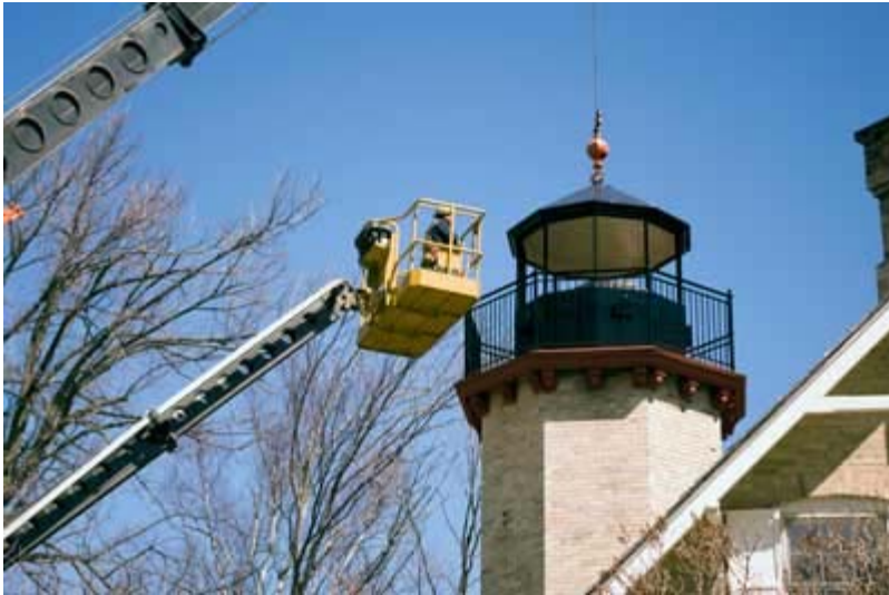
The tower looks exactly as it did over 100 years ago. Only glass panels and a top ornament are left to be installed.
