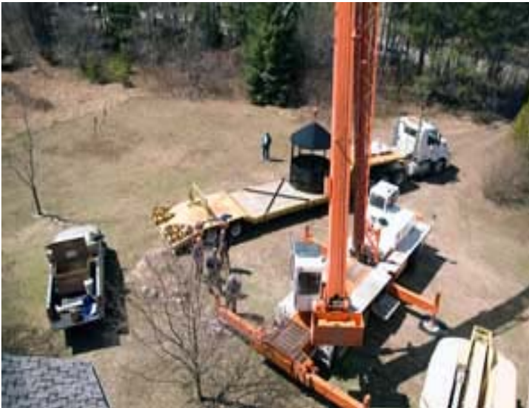
Scene of the installation of a new Lantern and Railing, viewed from atop McGulpin Point Lighthouse
