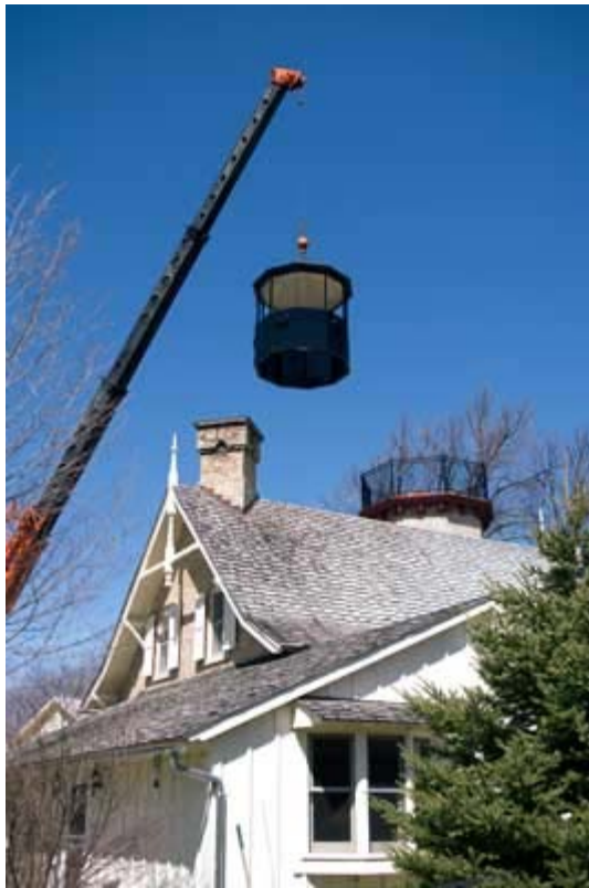
After the railing is secured, the lantern itself is lifted to the top of the tower.
