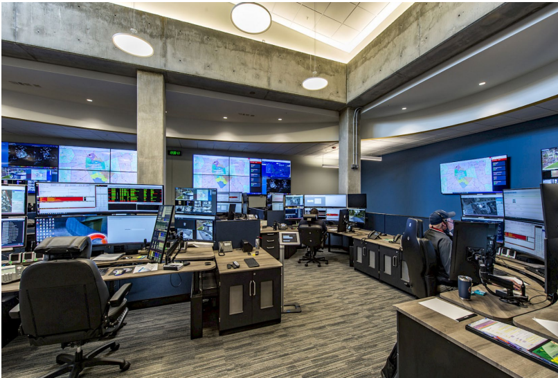
Photo: Inside the SEMRECC 911 Dispatch Center
