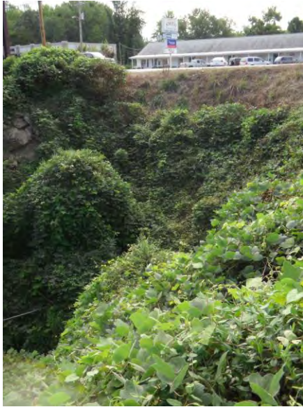
Brushy Creek is piped under Highway 123
