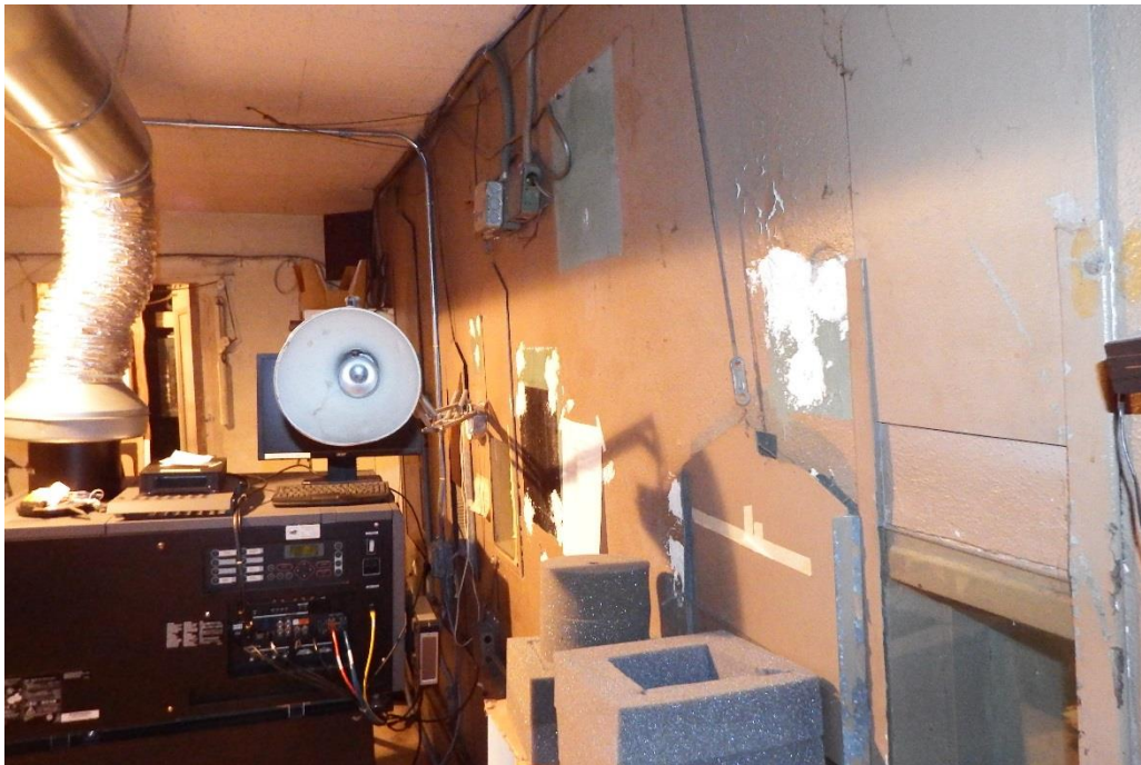
Figure 14: Current projection booth interior, looking north, note metal drop shields over lights (Jacobsen, 2020)
