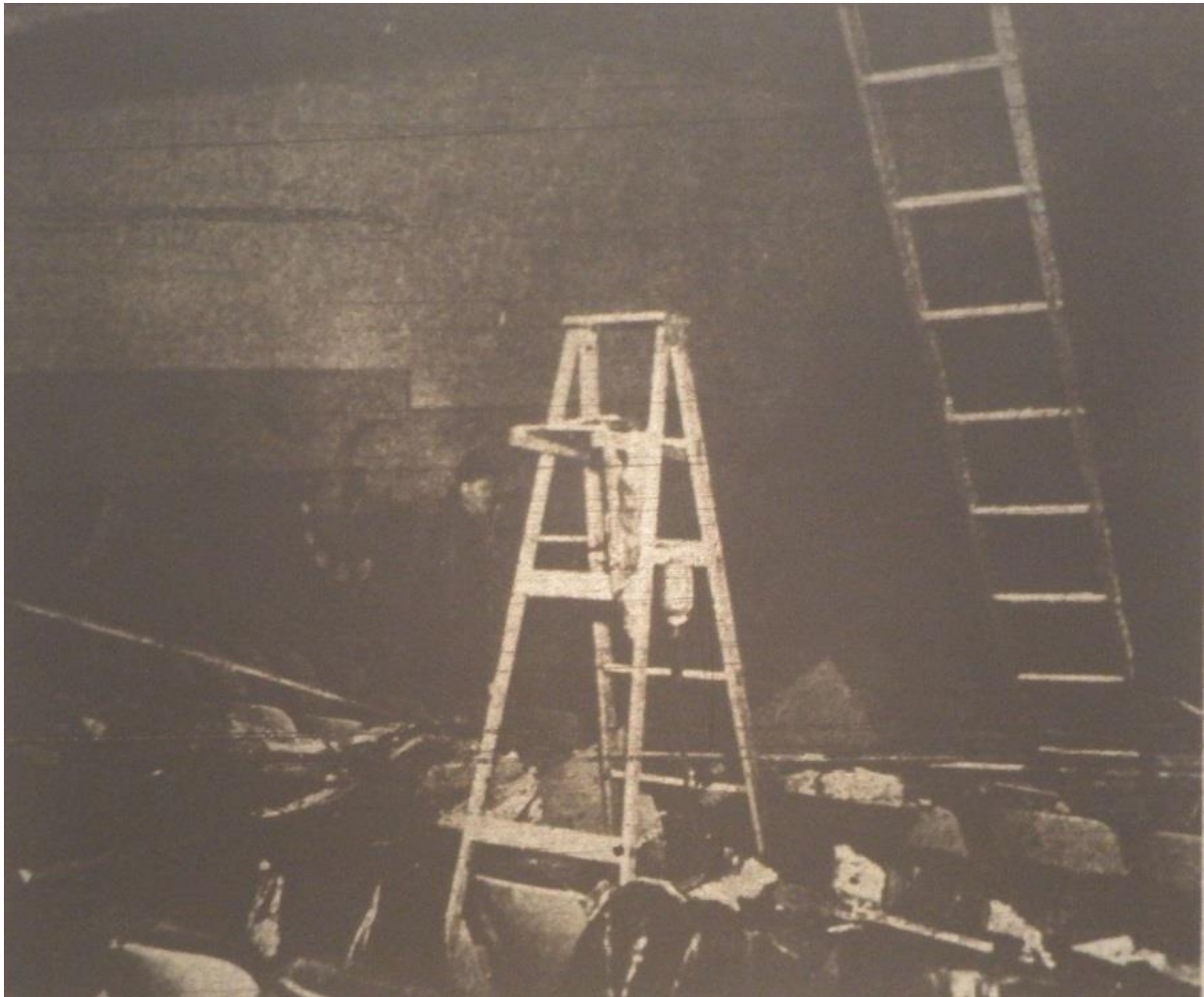
Figure 92: Fire damage in the east auditorium, looking northeast (Des Moines Register , January 23, 1958)
