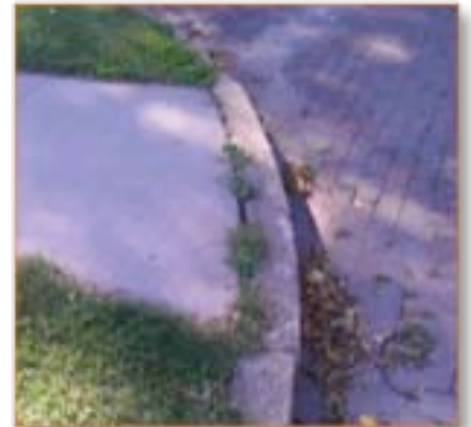
Figure 15. No curb cut
