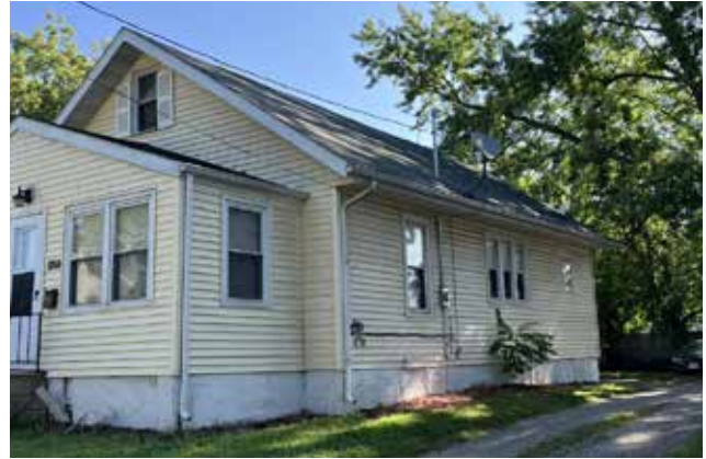
Figure 18. A "before" photo of an ION project to repair a foundation and roof. (Source: City of Des Moines)
