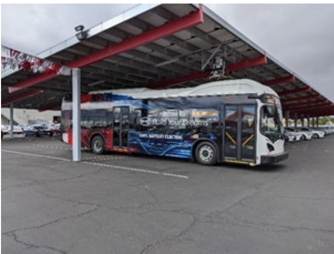
Figure 6. In-Depot Overhead Charging Example (Source: CALSTART)
