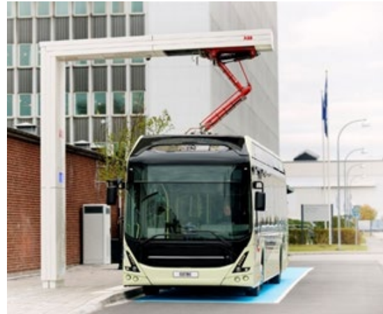
Figure 8. On-route Overhead Charging (Source: ABB)
