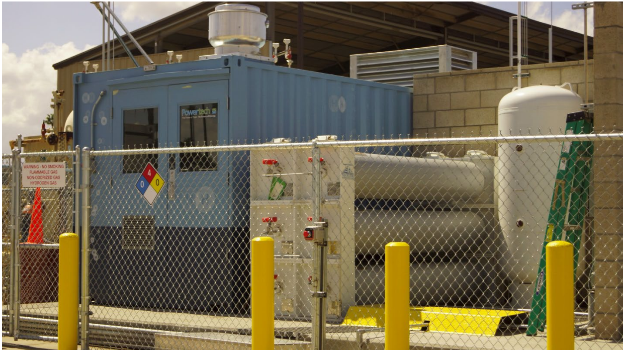
Figure 1: Powertech fuel processing module and high-pressure storage at the Riverside hydrogen refueling station. Image Credit: Hydrogen Ventures.
