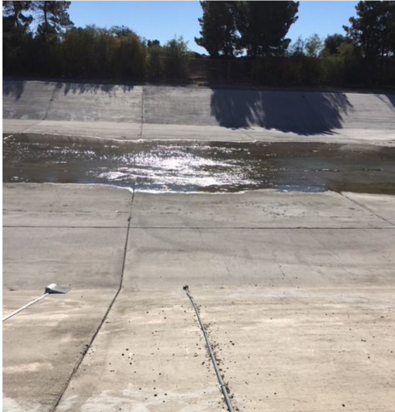
Figure 2-4. Conduit and strainer during dry weather at Club at Sunrise monitoring station
