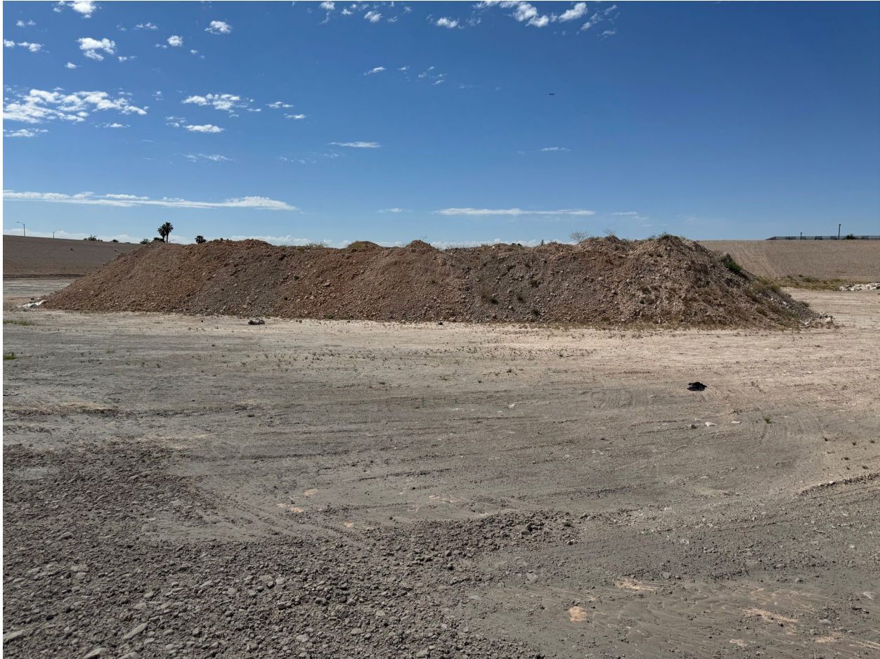
Figure 6. Sediment stockpiled for removal at Oakey Detention Basin
