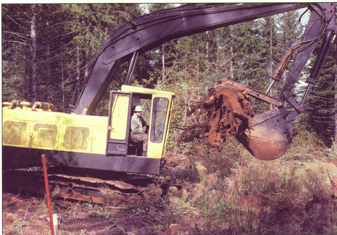
Figure 25—A large excavator with a standard bucket and an optional gripping thumb can be used effectively for stump removal.
