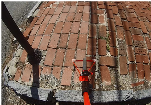
Example of Sidewalk with No Ramp
