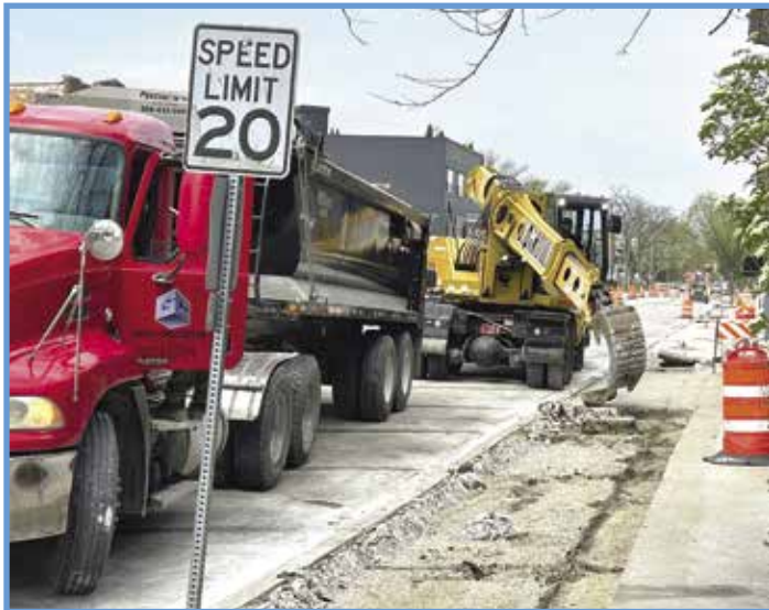
An excavator removes concrete sidewalk from the parkway area on the east side of the 3700 block of Grand Boulevard in preparation for the installation of a new sidewalk, decorative brick pavers, street lights, trees and a seat wall at the corner of Grand and Prairie.
