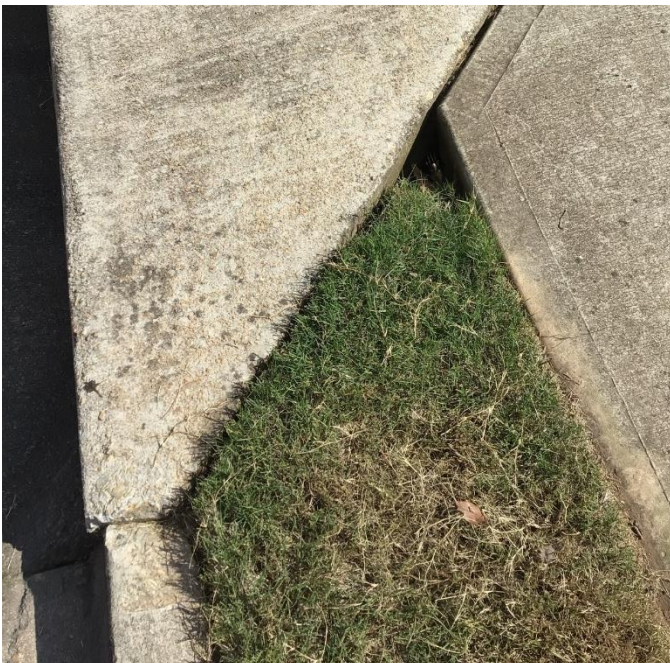
Figure 3.11 7370 Silk Tree Pointe – Void at Catch Basin
