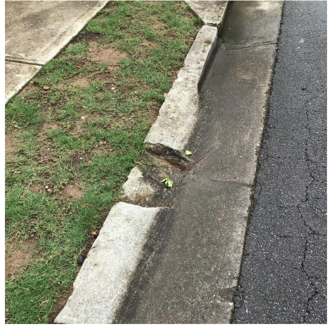
Figure 1.7 2073 Democracy Drive – Broken Curb
