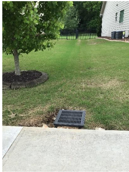
Figure 5.14 6225-6229 Riverview Parkway – Drain Box and Voids
