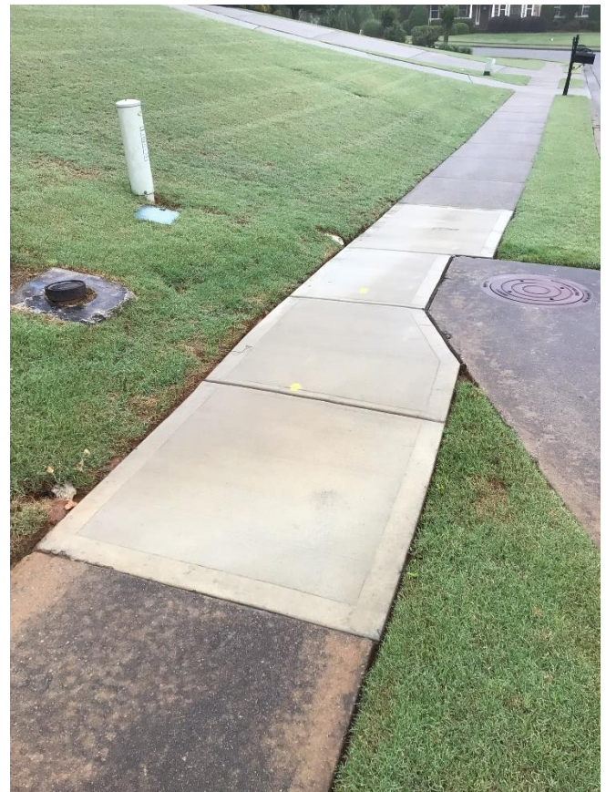
Figure 1.3 2436 Commissioner Cove – Void at Catch Basin
