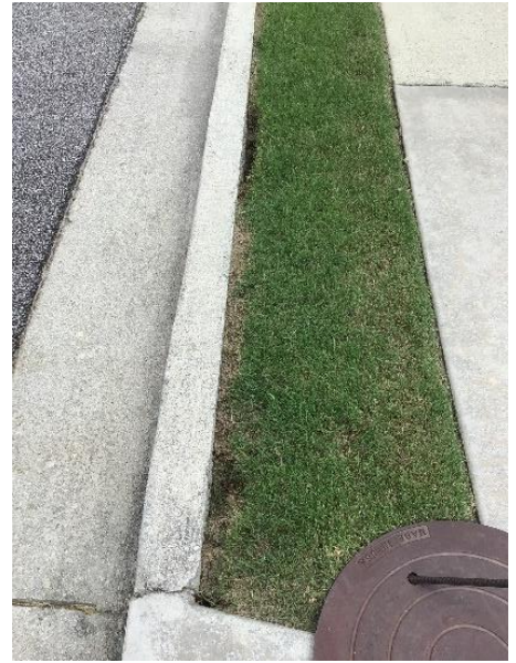
Figure 5.18 6237-6241 Riverview Parkway – Voids
