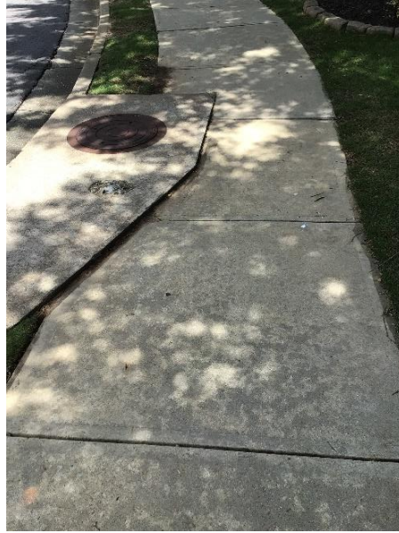
Figure 5.21 Roundabout near Entrance – Settled Sidewalk
