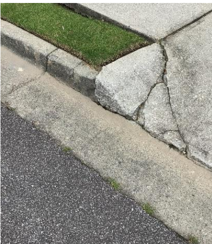
Figure 5.3: 5767 Berkshire Trace – Damaged Driveway
