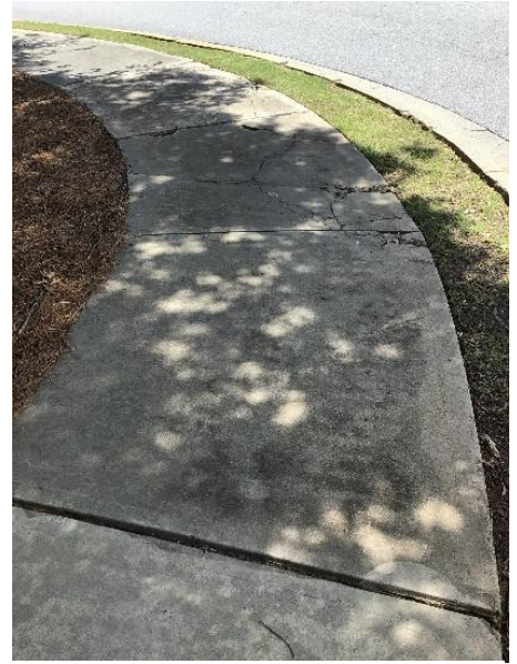
Figure 5.22 Roundabout near Entrance – Damaged Sidewalk
