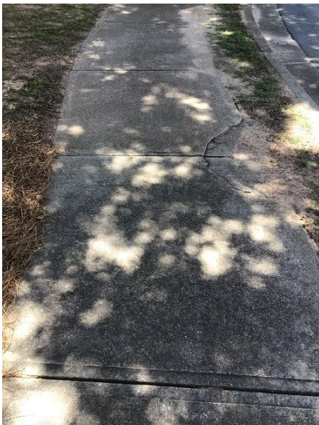
Figure 5.23 Roundabout near Exit – Damaged Sidewalk
