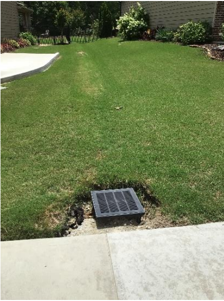
Figure 5.16 6237-6241 Riverview Parkway – Drain Box and Voids
