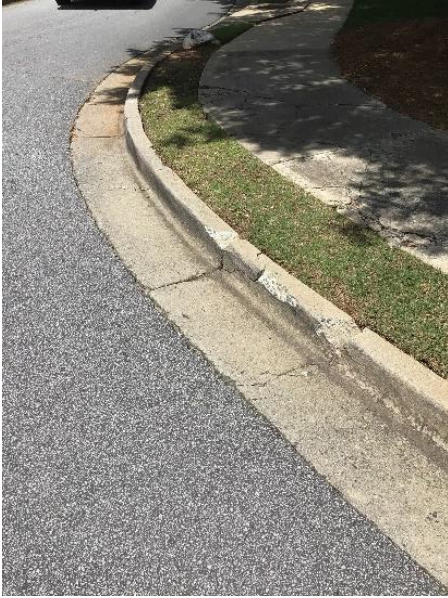
Figure 5.20 Roundabout near Entrance – Damaged Curb and Gutter
