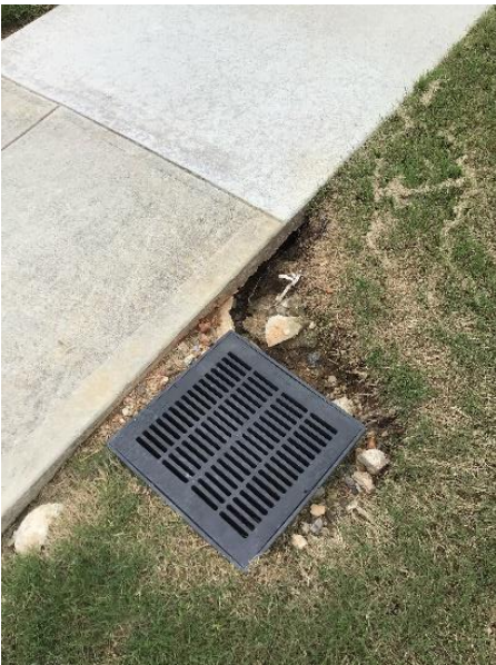
Figure 5.13 6225-6229 Riverview Parkway – Drain Box and Voids
