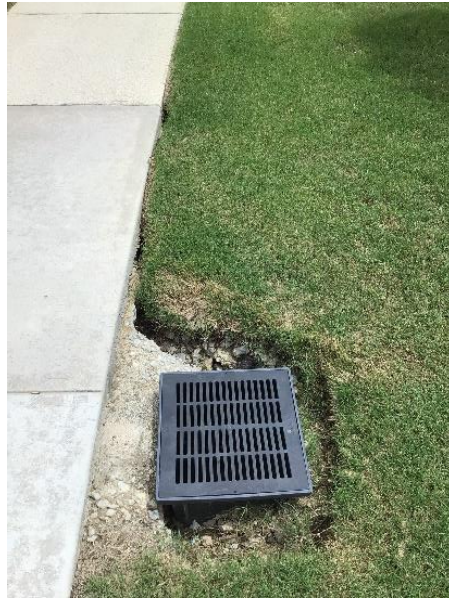
Figure 5.17 6237-6241 Riverview Parkway – Drain Box and Voids
