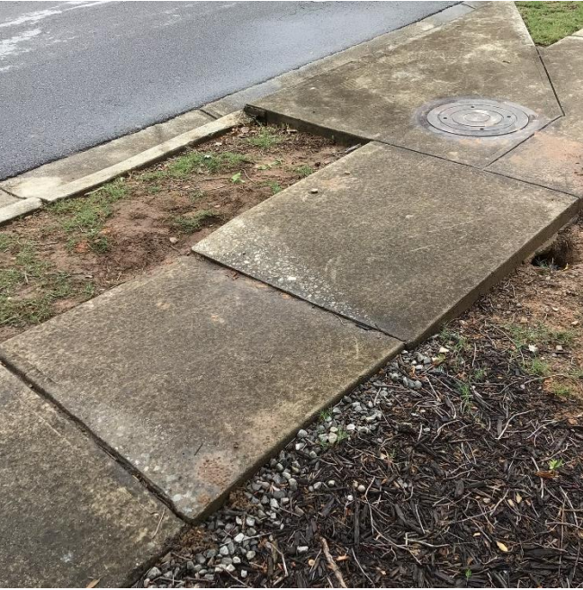
Figure 1.6 2073 Democracy Drive – Settled Sidewalk
