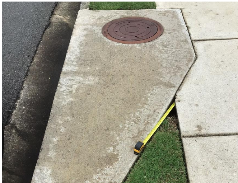
Figure 1.8 2207 Democracy – Void at Catch Basin
