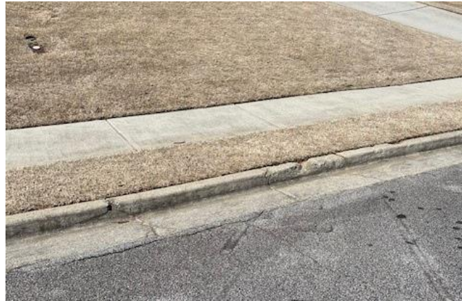
Figure 1.1 2436 Commissioner Cove Street View – Damaged Curb and Gutter
