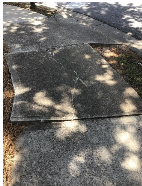
Figure 5.24 Roundabout near Exit – Damaged Sidewalk
