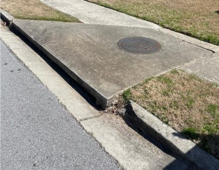
Figure 1.14 2144 Independence Lane – Damaged Curb
