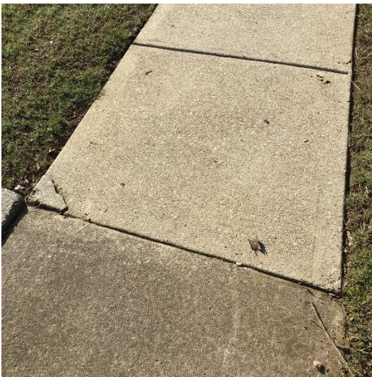
Figure 2.2 852 New Liberty Way – Settled Sidewalk
