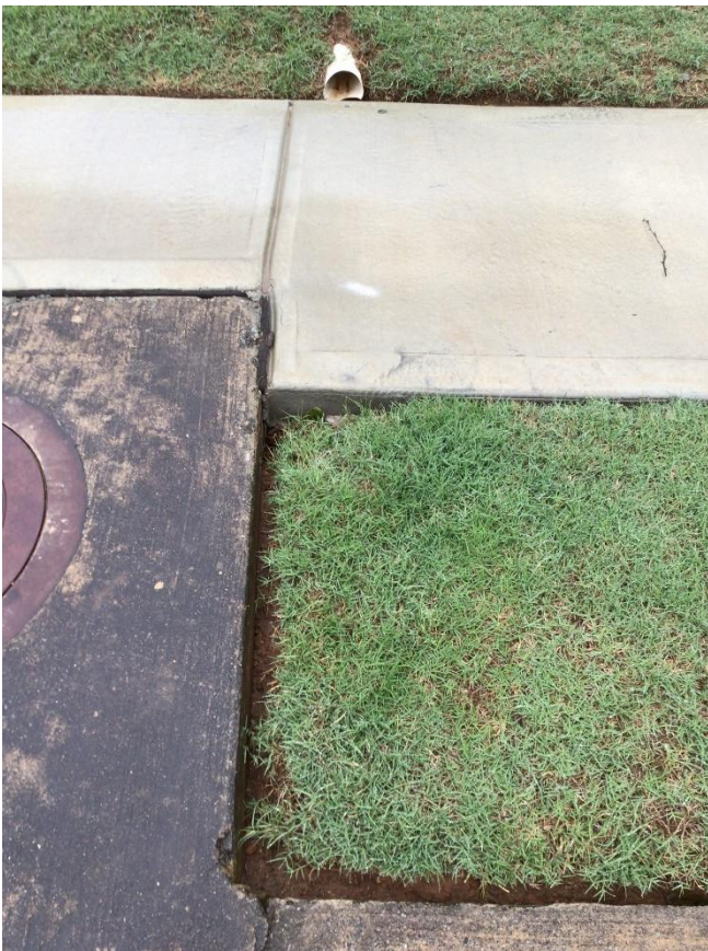
Figure 1.2 2436 Commissioner Cove – Void at Catch Basin; Location of Proposed Concrete
