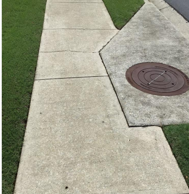
Figure 1.17 2955 Legislative Lane – Sidewalk damage
