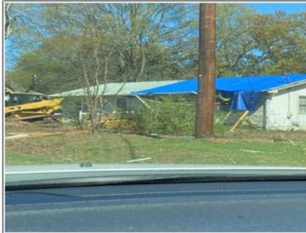
This home sustained damage in the tornado.
