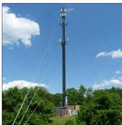
GUYED LATTICE TOWER
