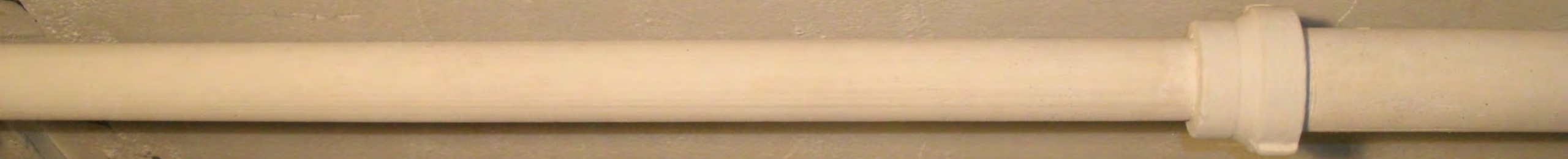
Original Electrical Wooden Raceway
