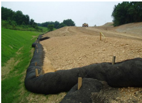
Ends of this filter sock are upturned to impound runoff. Stakes are placed in the center of the socks.
