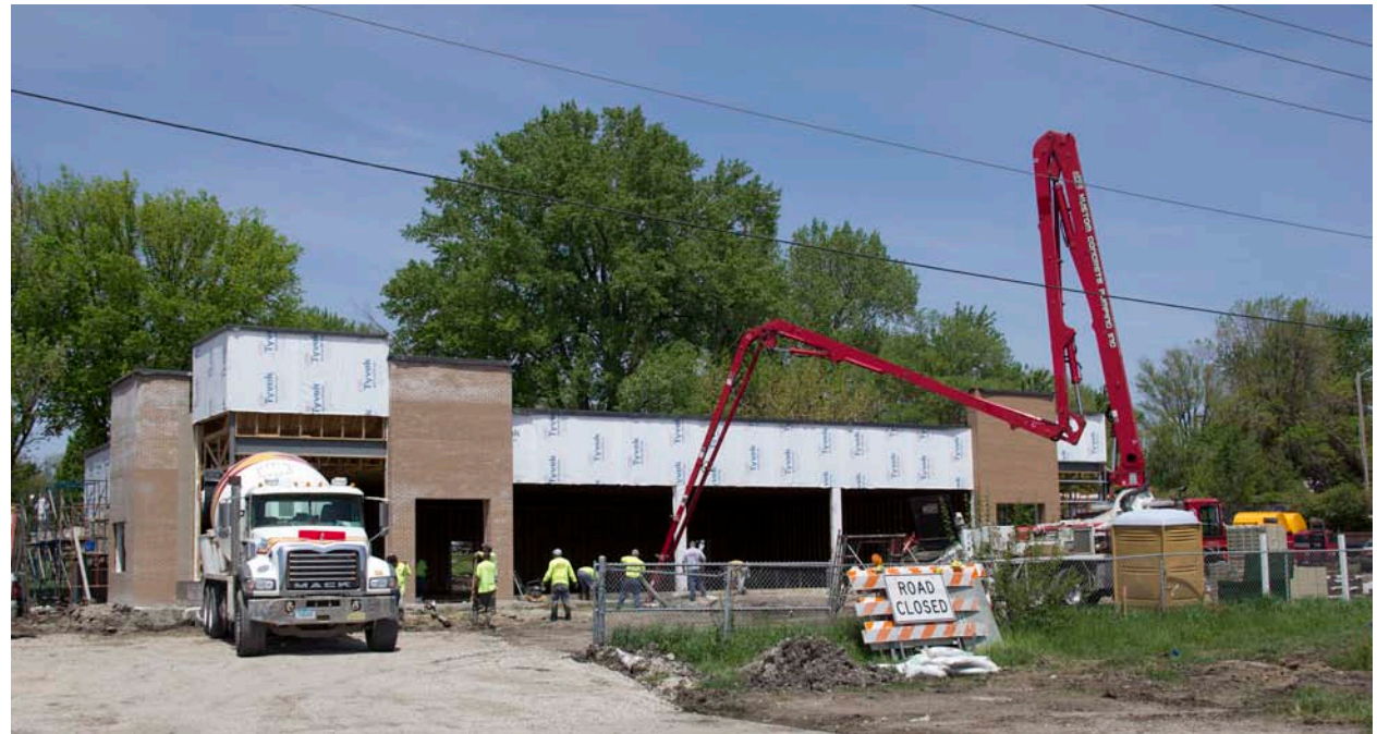
Above: A new commercial building under construction on 8th Street in Altoona.
