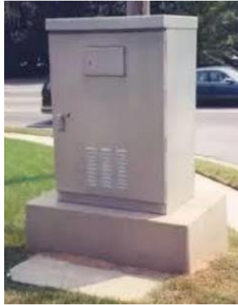
(Example of a Traffic Box )
