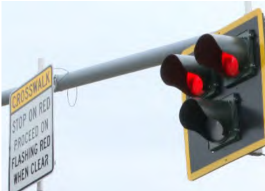
PEDESTRIAN HYBRID BEACON LIGHT + SIGN
