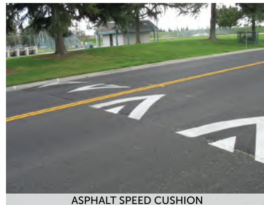
ASPHALT SPEED CUSHION
